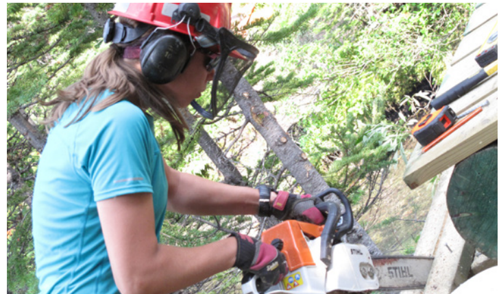
A BTFR trail crew member putting on the finishing touches to the Lyaill Creek bridge
