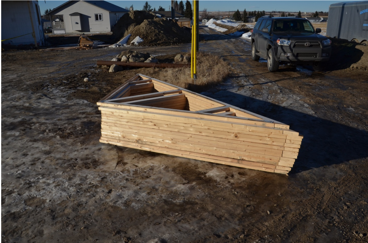
Figure 3. Trusses from the incident
