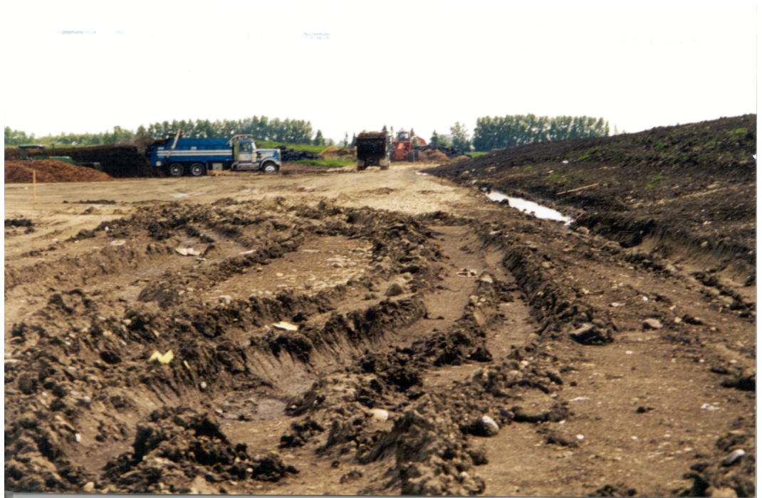
Figure 2-1: Compacted clay pad with ruts and leachate accumulation arising from the use of equipment during heavy rainfall.
