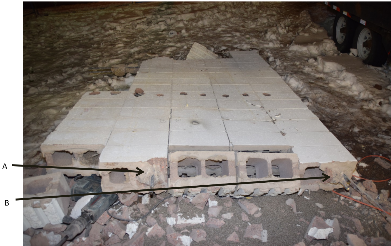
Figure 6. Steel rebar encased in concrete within the exterior cinderblock wall.
