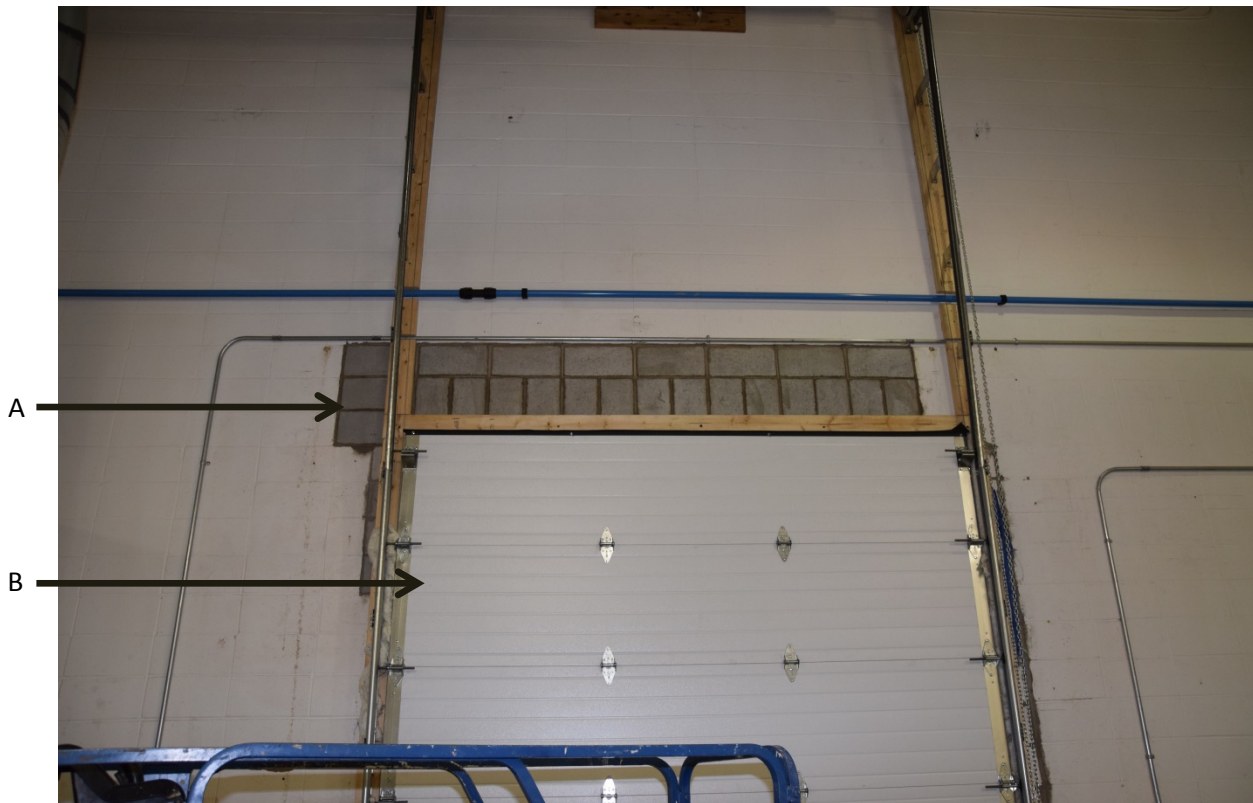
Figure 1. Cinderblock lintel construction and new bay door installation. View from inside 601-28 th St NE commercial building.
