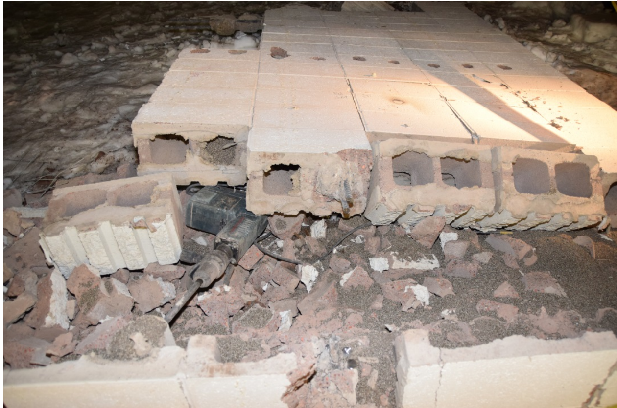
Figure 2. Shows a Bosch electric demolition hammer under collapsed block wall.
