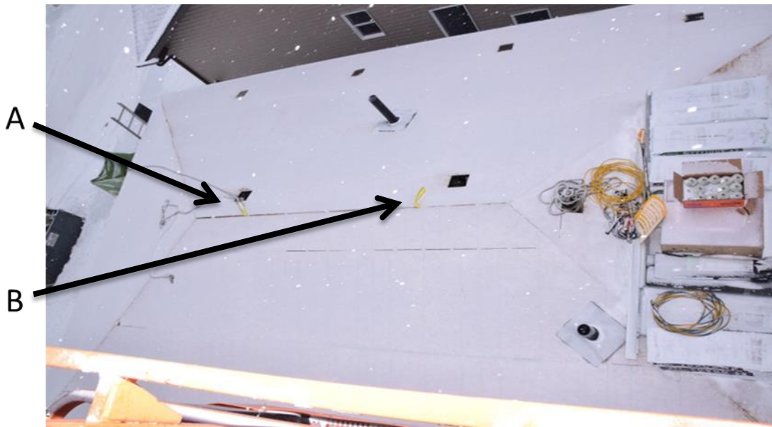
Figure 1 - West sling anchor (A) with two lifelines attached to it. The materials on the right side of the photo included the life line worker one had been using and the extension cord which became tangled. The site had been cleaned up prior to OHS arrival. East Sling Anchor (B) - anchor worker one had been connected to prior to the incident.
