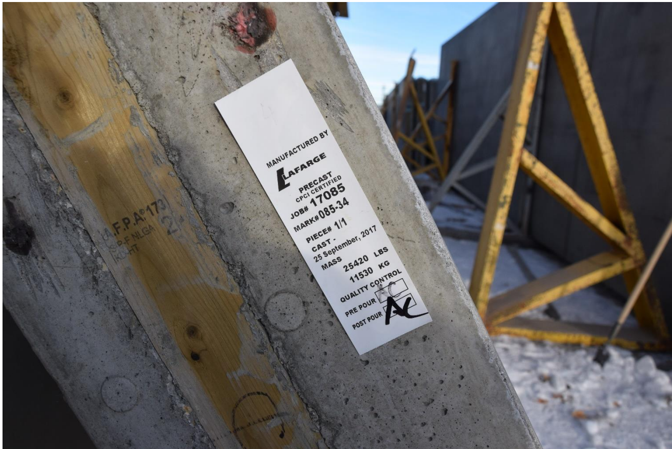
Figure 4. Label on Insulcore Panel 085-34 that tipped and fell
