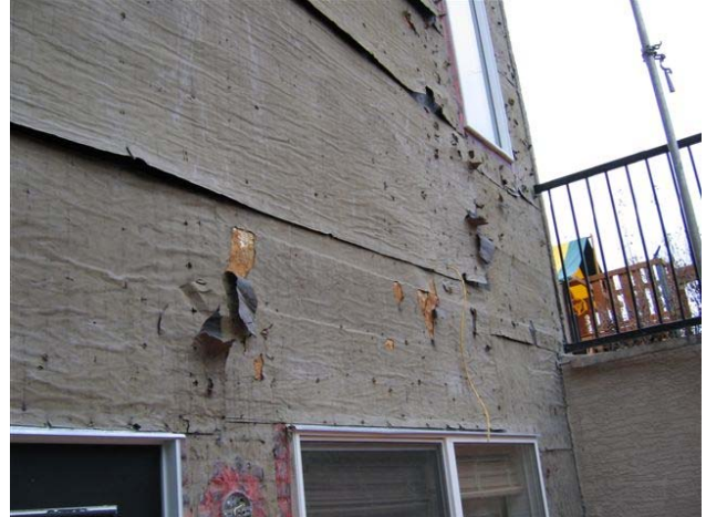
Damaged building paper due to prolonged exposed to weather
