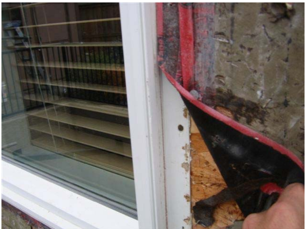
Improperly installed window
