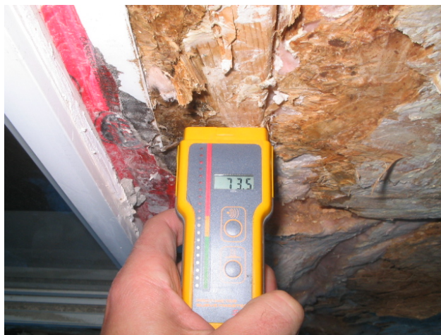
Moisture content of 73.5% should be less than 19%
