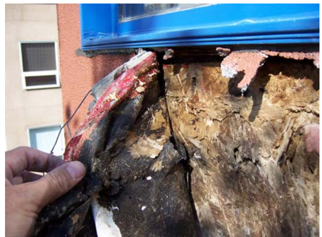
Moisture damage under exterior finish
