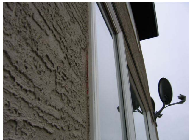
Improper stucco thickness
