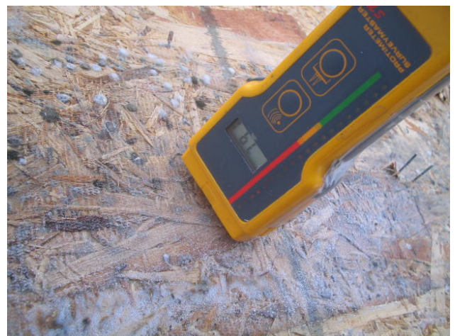
Moisture content of 79% should be less than 19% (mould growth in background)
