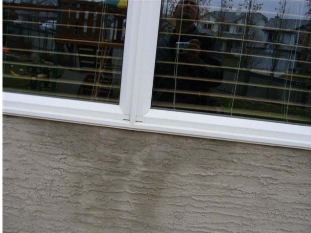
Water damage beneath window sill
