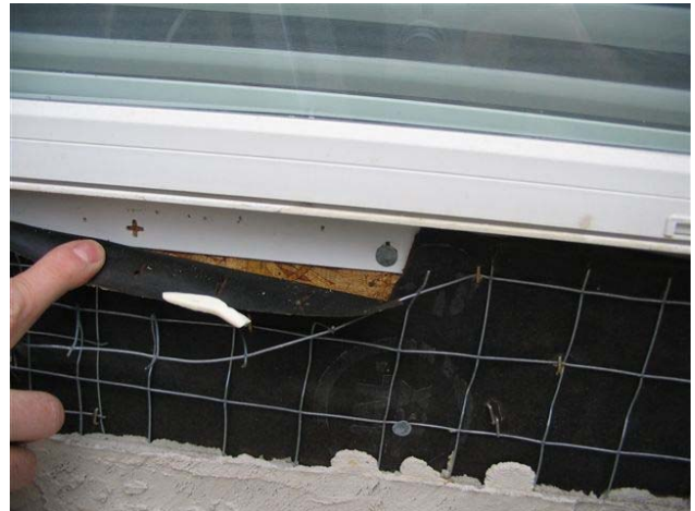
Window flange not nailed properly
