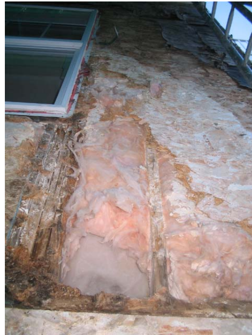
Damaged studs and exterior sheathing
