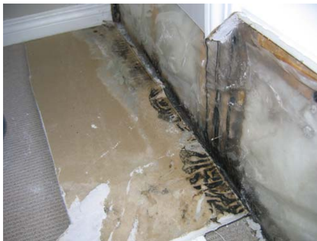
Interior drywall with mould growth
