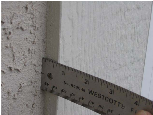
Improper stucco thickness
