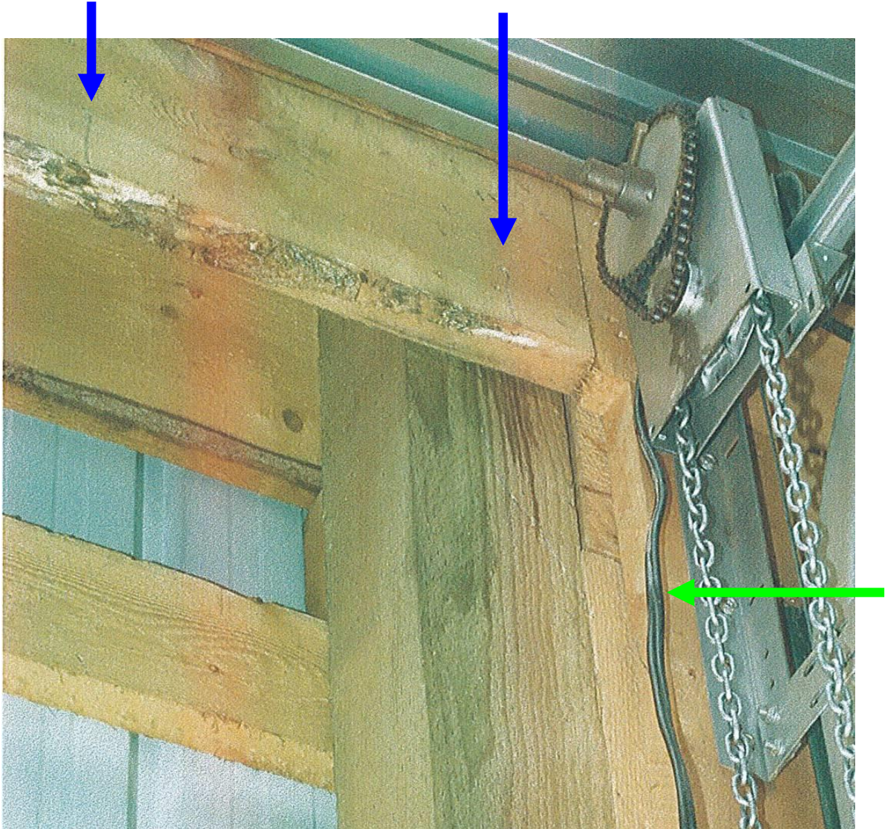
Photograph 5 – Shows the electrical wire running up and over the overhead door. The blue arrows point to the marks on the upper cross member. The green arrow points to the electrical wire.
