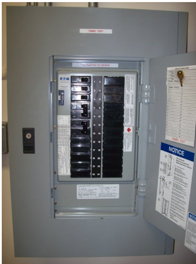
Cutler hammer panelboard
