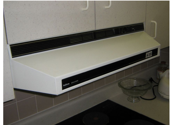
Existing range hood.
