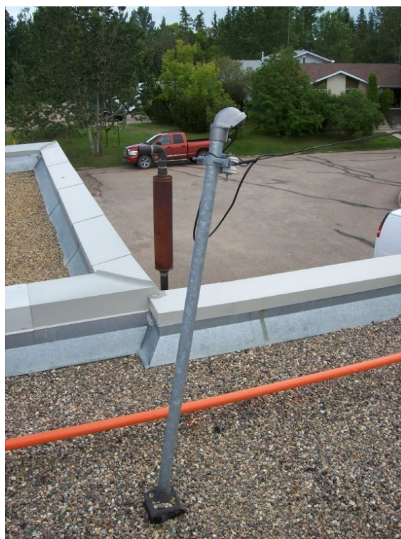
Crooked CATV service mast
