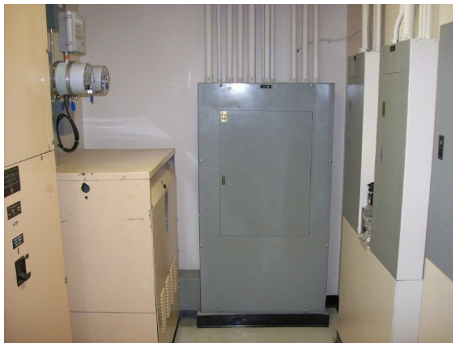
Typical floor mounted transformer
