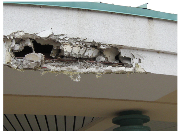
Damaged stucco at fascia of pavilion.
