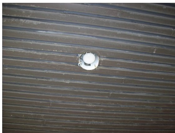
Missing trim on downlight
