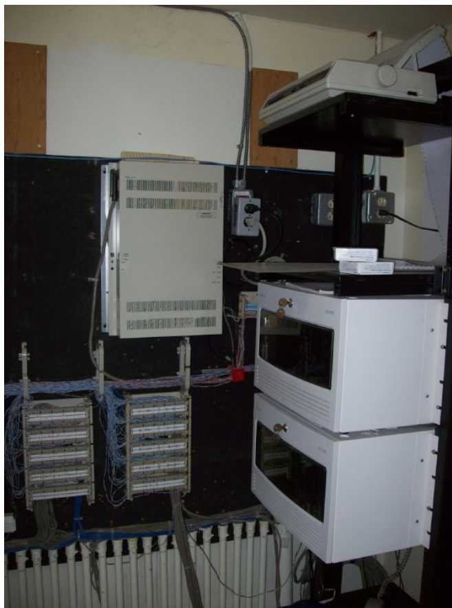
The Mitel PBX equipment in the telephone room
