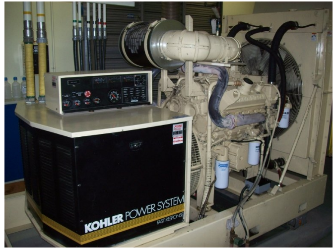
250KW Kohler/Detroit Diesel Genset.
