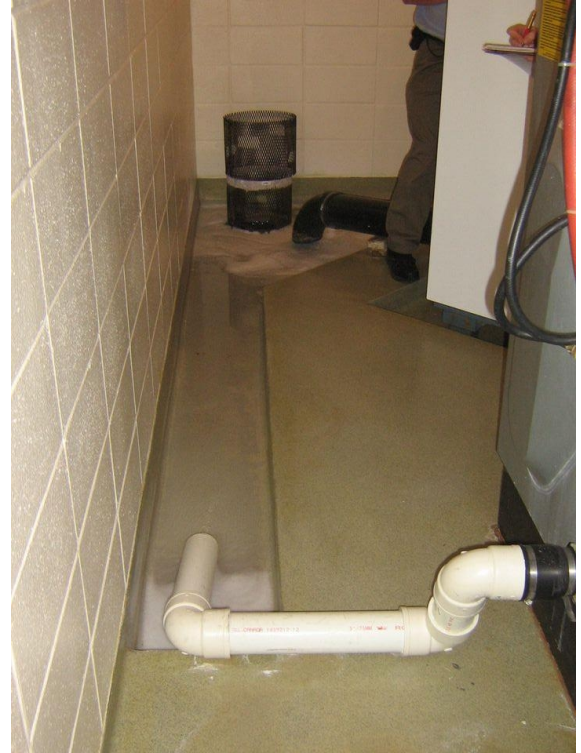
Washing machine drains.
