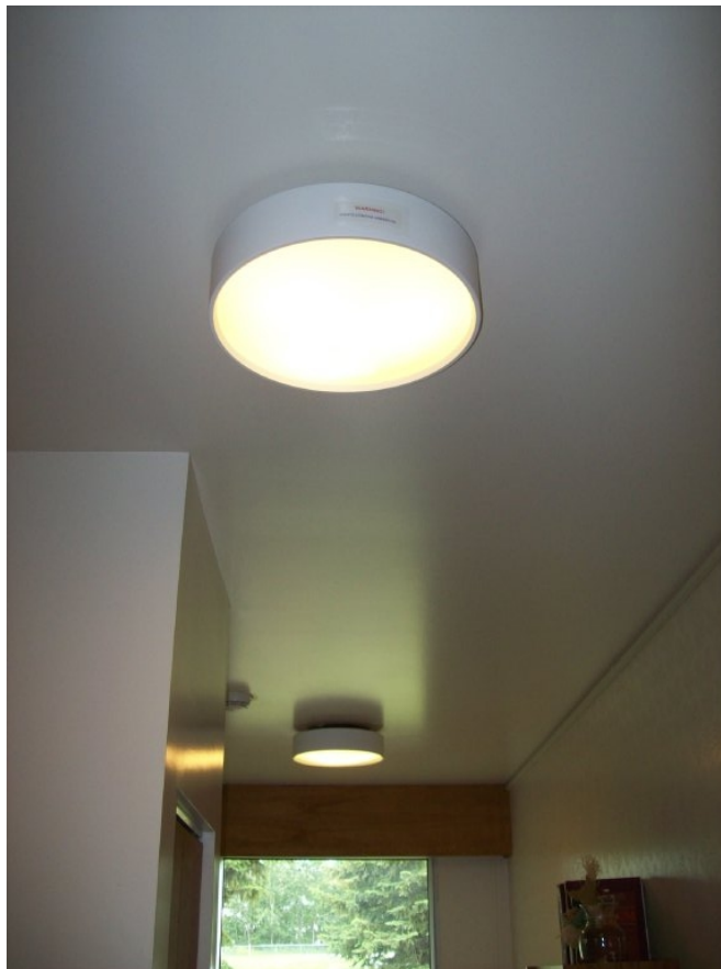
Incandescent drum lights that contain asbestos
