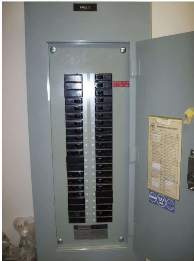
Typical Westinghouse branch circuit panel
