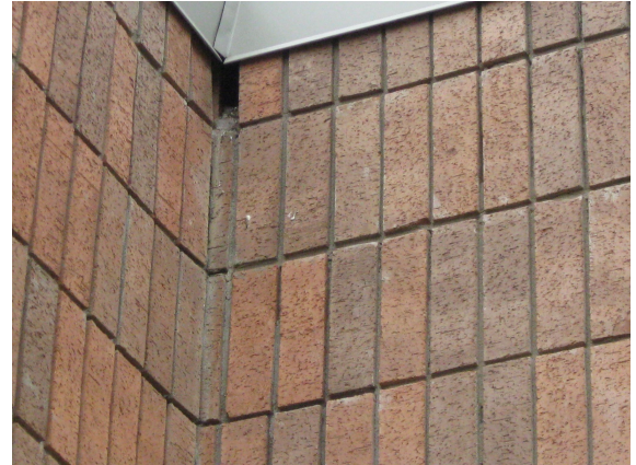
Missing brick at soffit.
