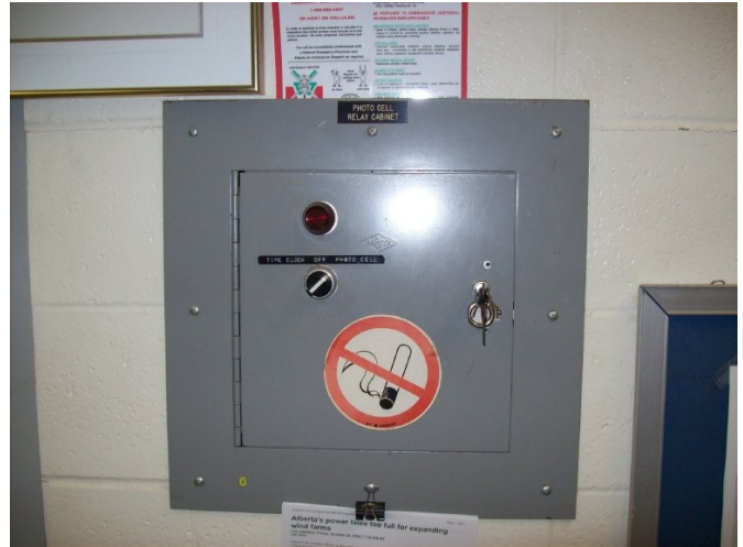
Exterior lighting relay control cabinet
