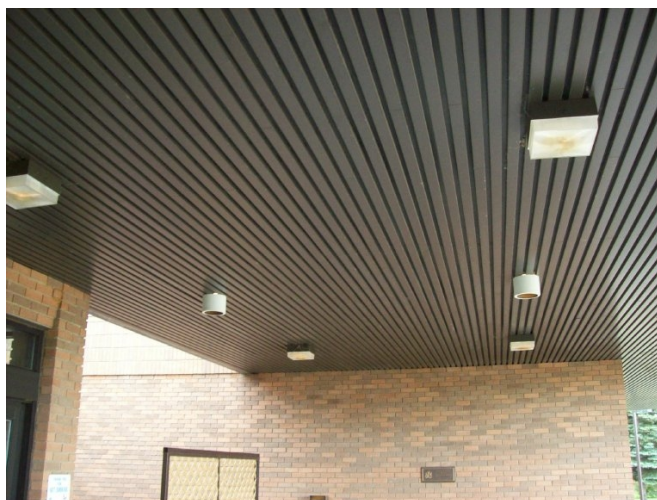
HPS Canopy fixtures.
