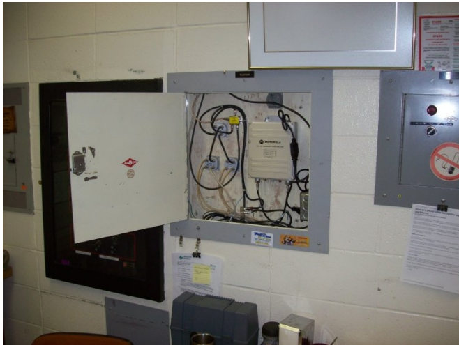
The main CATV demarcation
