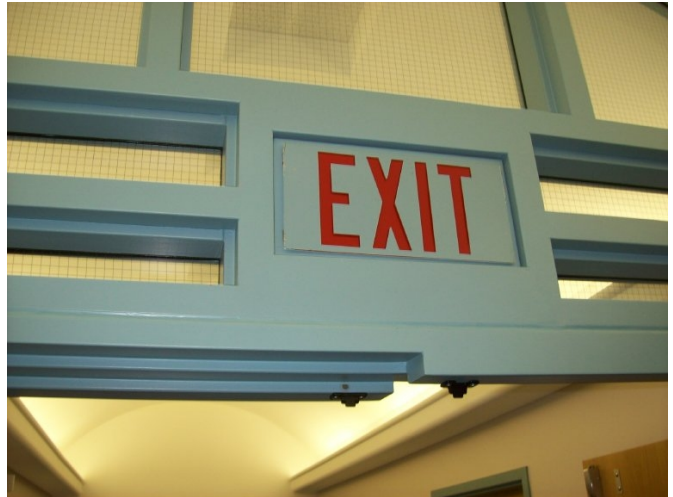
Recessed exit sign in Parkview L.T.C.
