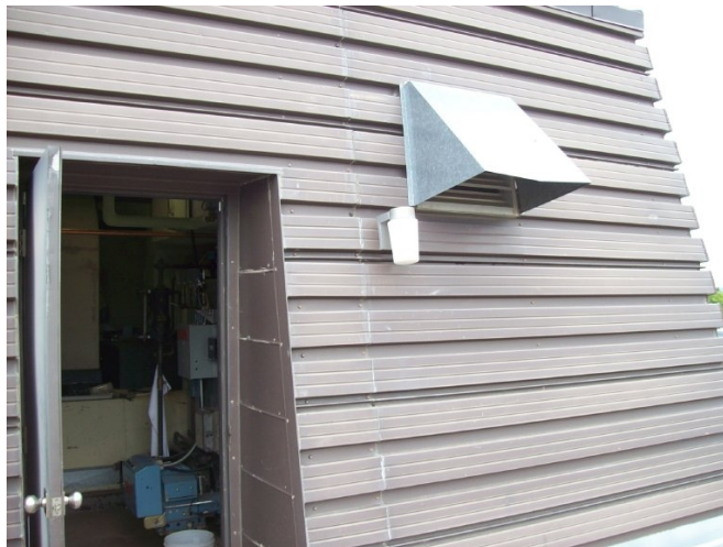
Exterior incandescent fixture at roof
