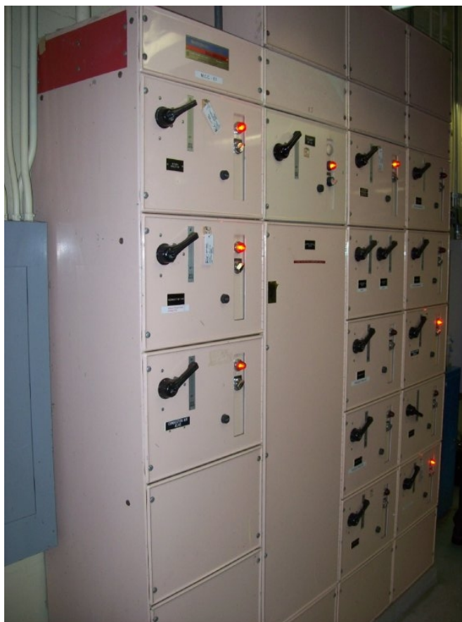
Westinghouse 4 section MCC
