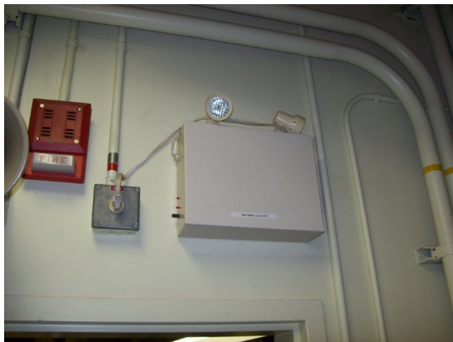
Emergency battery pack in generator room
