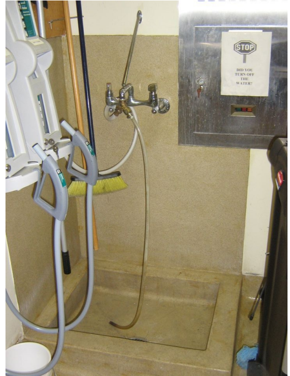
Isolation panel located at the mop sink
