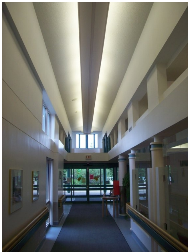
Typical fluoescent cove lighting in main corridors.
