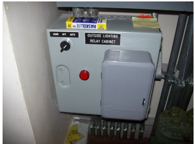
Exterior lighting relay cabinet and timeclock
