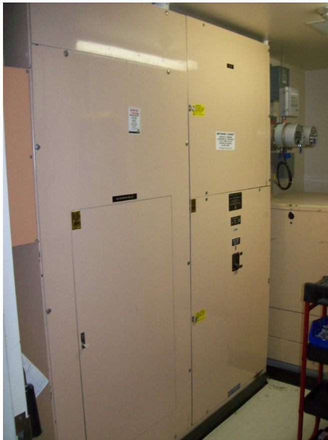
The Westinghouse 1200A 120/208V 3ph 4w main distribution
