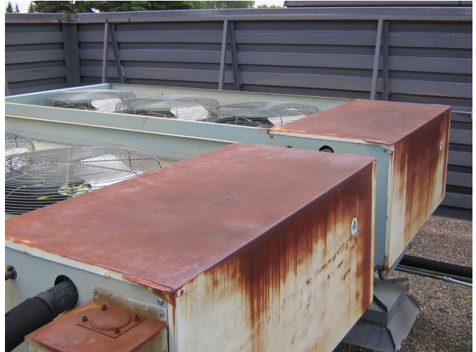
Rusted condensing units.
