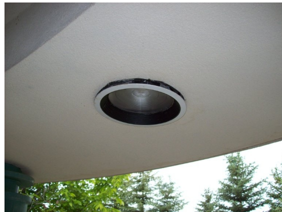
Trims separating from downlights.
