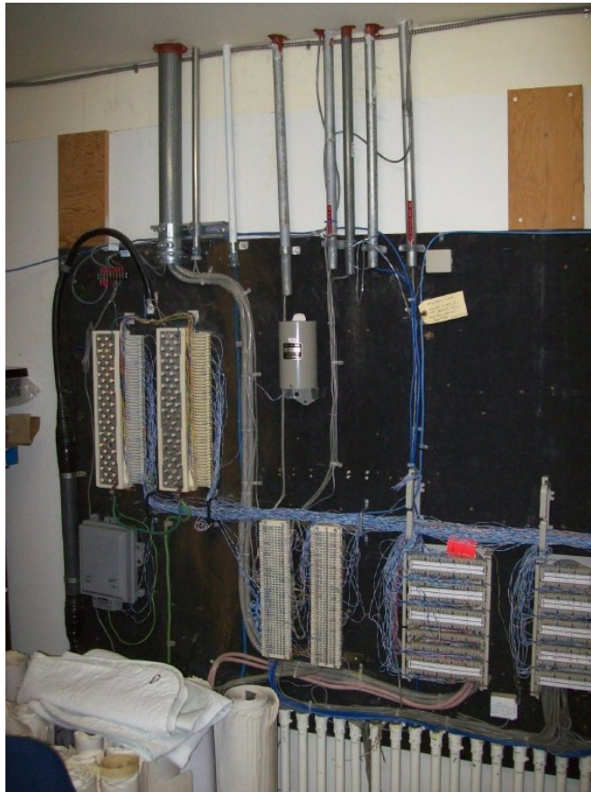
The main telephone demarcation
