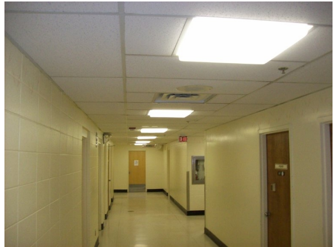
Drop lens fluorescent fixtures in health centre corridor.
