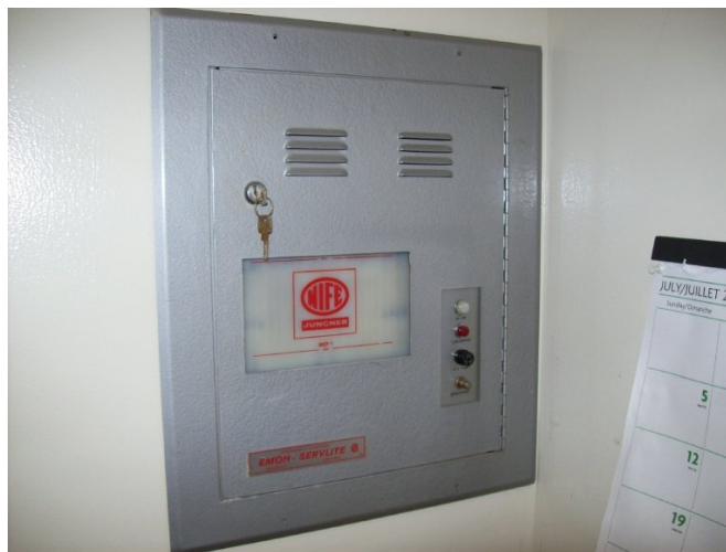
O.R. Area emergency lighting backup panel
