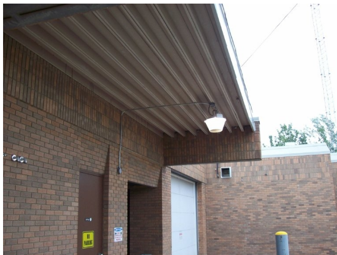
Low bay fixture at maintenance entry
