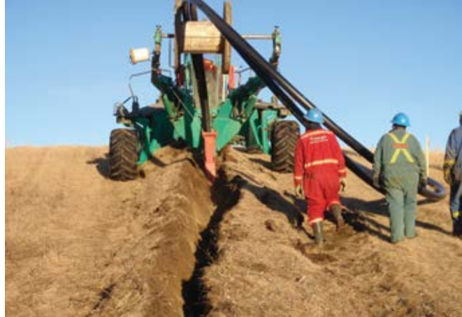
Spiderplow pipeline installation Northern Fescue NSR during dry conditions in November (Desserud 2009)
