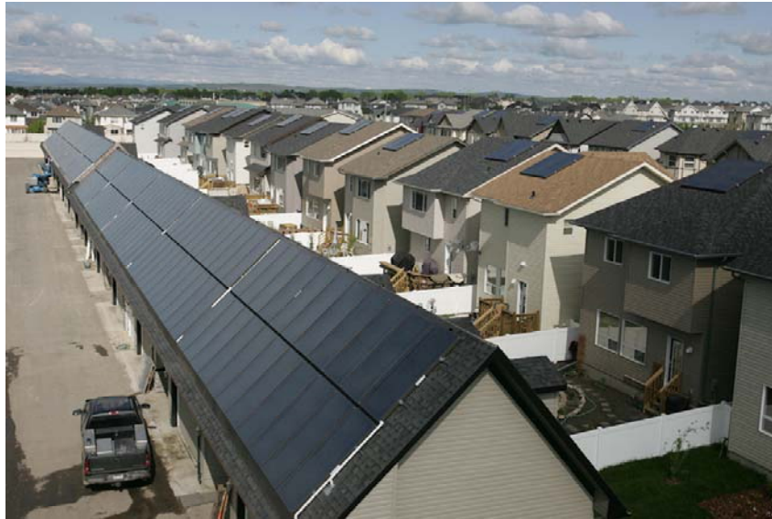
Figure 5.51 Solar Thermal – Drake Landing, Okotoks, Alberta
