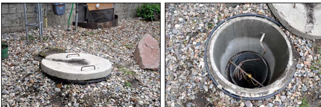
Figure 11: Well 4 located on Site 1.
