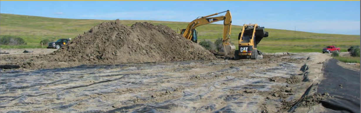
Use of Barrier Fabric to Conserve Surface Vegetation. Trained Operators with Experience are Key to Success!
