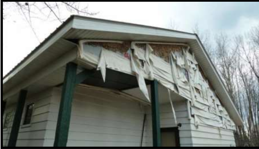
Figure 122 – Melted vinyl siding illustrating the potential for it to be blown away by the wind if ignited, thus spreading fire downwind.
