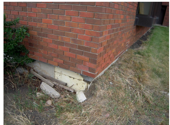
Damaged asbestos board
