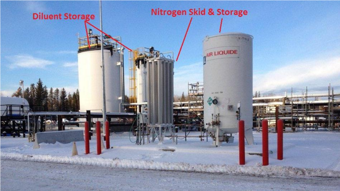
Figure 12: N2 and Diluent Storage
