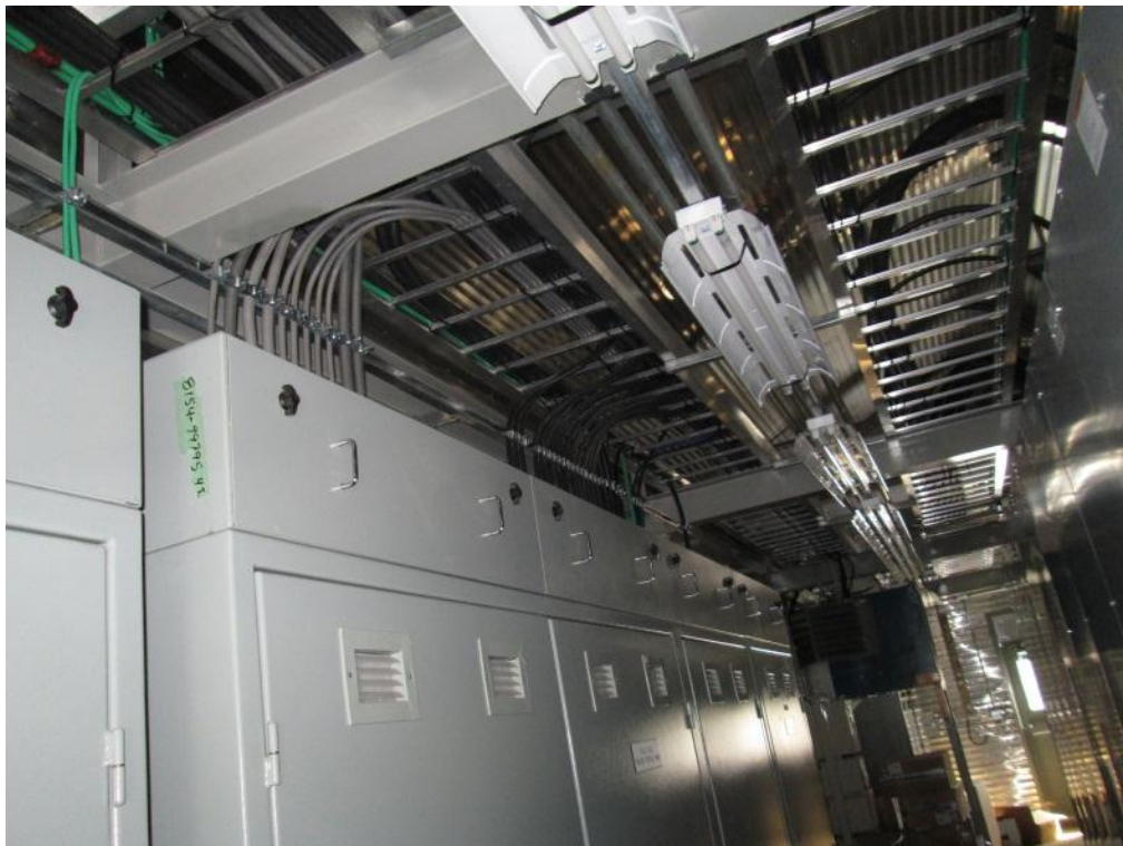
Figure 10: Interior of MCC Building
