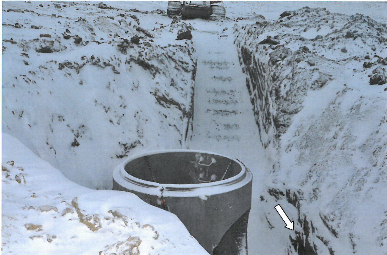
Photograph # 5 A portion of the straight cut wall that Worker 1 [REDACTED] was crushed against is identified by the arrow. A portion of the three legged chain sling used to attach the vertical manhole portion to the excavator is visible draped over the top of the vertical manhole portion.
