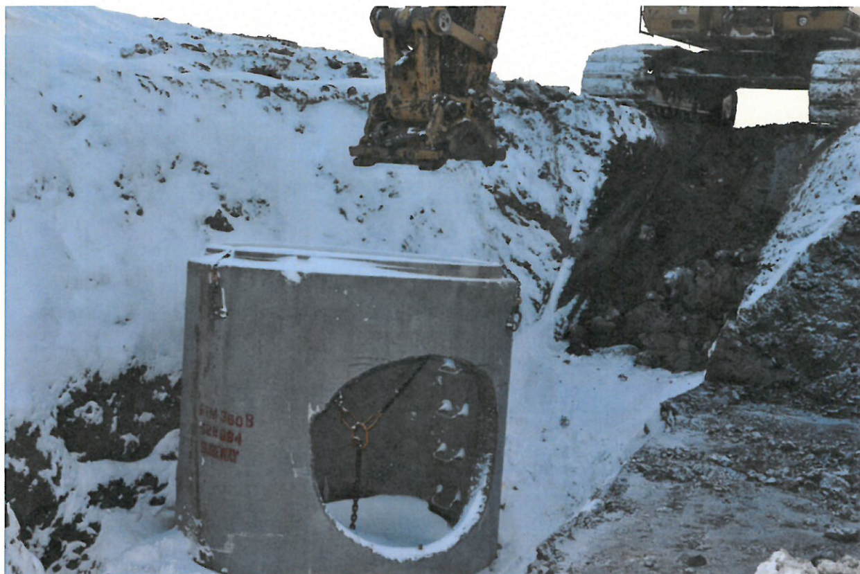
Photograph # 8 Shows a part of the chain sling inside the vertical manhole portion which struck and crushed Worker 1 [REDACTED]. The circular cut out shown in the vertical manhole portion was intended to receive the horizontal storm drain sewer pipe.
