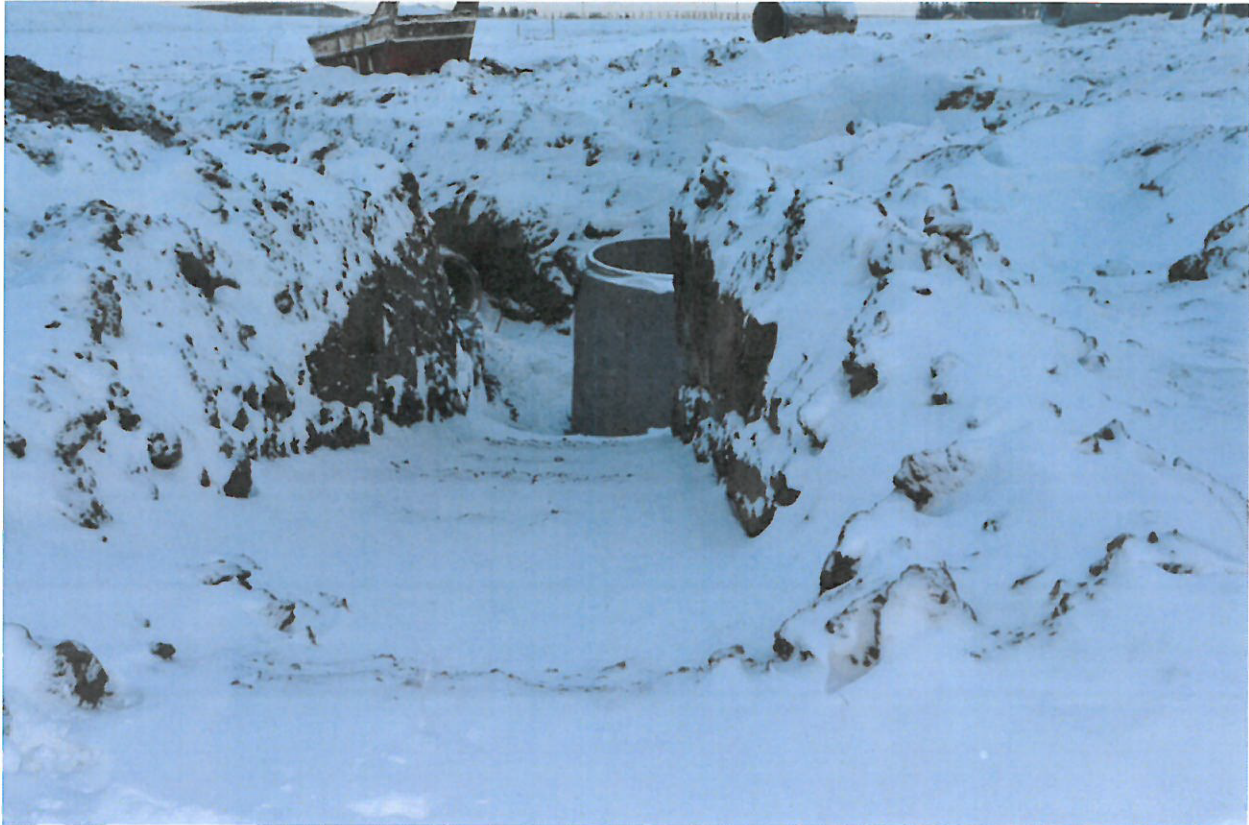
Photograph # 4 The trench that the excavator operator [REDACTED] dug immediately after the incident is shown in the foreground (south end) of this photograph. The vertical concrete manhole portion that struck and crushed Worker 1 [REDACTED] is also visible in the photograph.
