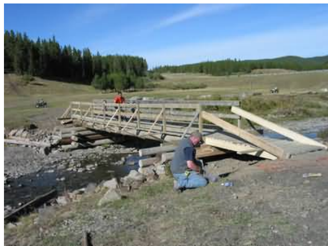
Volunteers building a bridge in the Ghost-Waiparous area, 2003 (Alberta United Recreationist Society photo)
