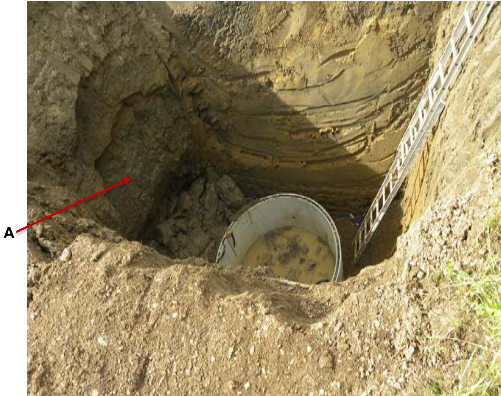
Figure 3. Looking into the excavation from the east side facing west. The picture was taken by the safety person at Tolko on September 1, 2020.
