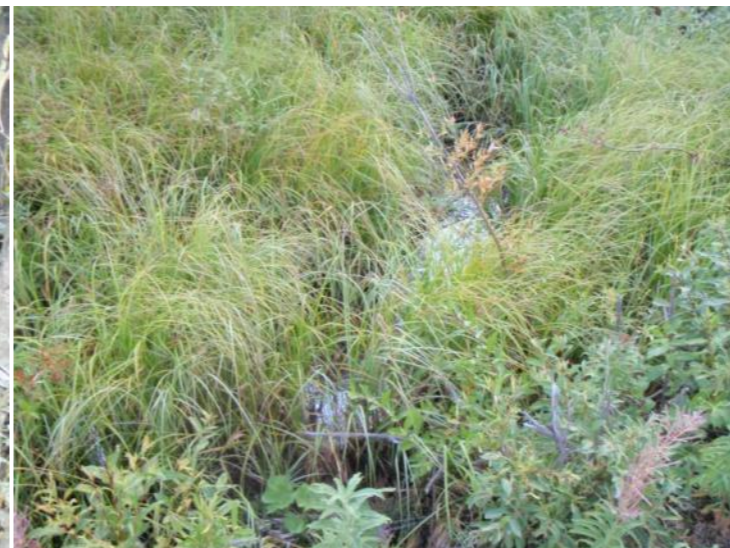
Photo 3: View of water pooled upstream of culvert (September 2011).
