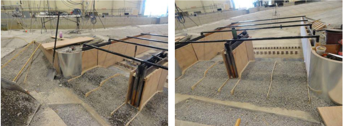
Figure 49. Installation of the narrower sidewalls, curved retaining walls, and preparations for pouring the concrete apron at the diversion.
