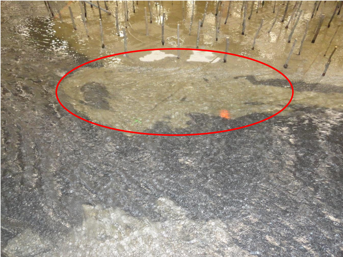
Figure 104. Erosion of sediment in secondary upstream flow channel (circled)
