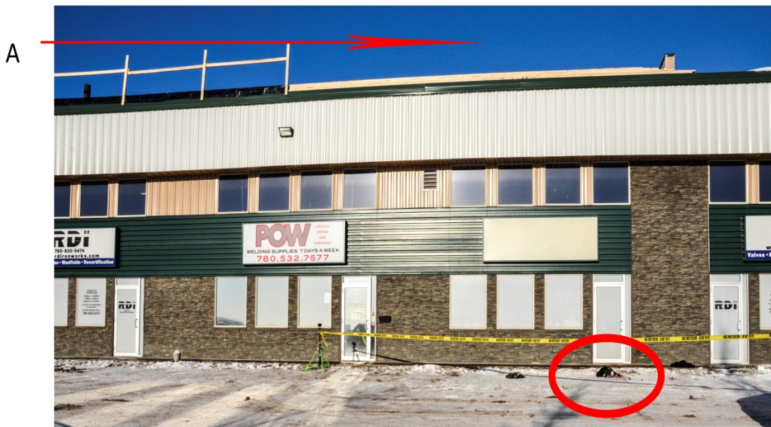
Figure 1. A indicates the unguarded south edge of the building where the worker fell from. The red circle indicates the location where the worker landed. (Photo taken by OHS)
