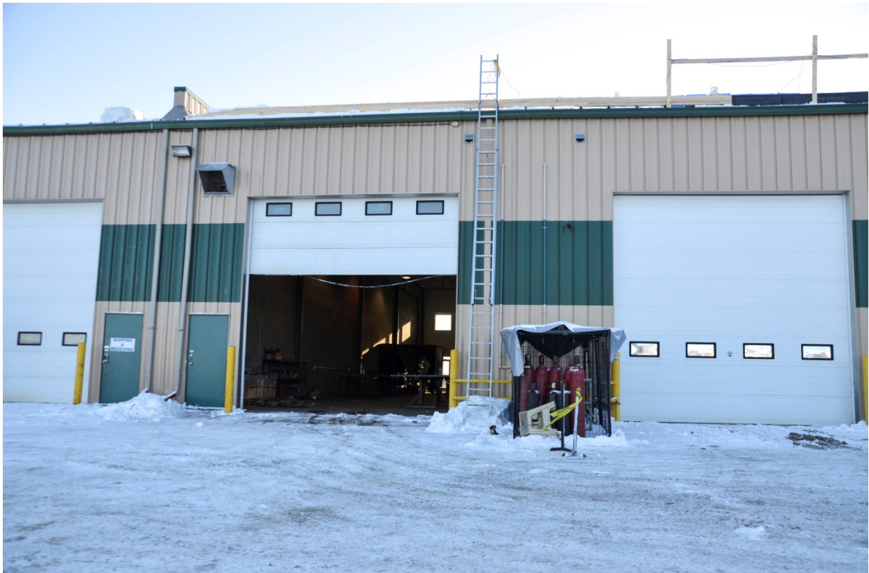
Figure 2. This is the north side of the building and shows the unguarded edge that measures 13.11 m in length. (Photo taken by OHS)
