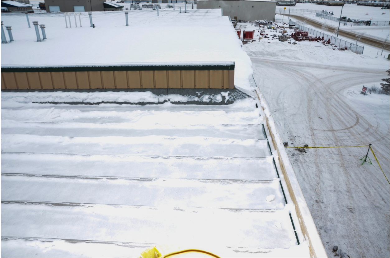
Figure 4. This is the south edge of the roof top where the worker fell from. The distance from the parapet to the ground was measured at 8.23 m. (Photo taken by OHS)
