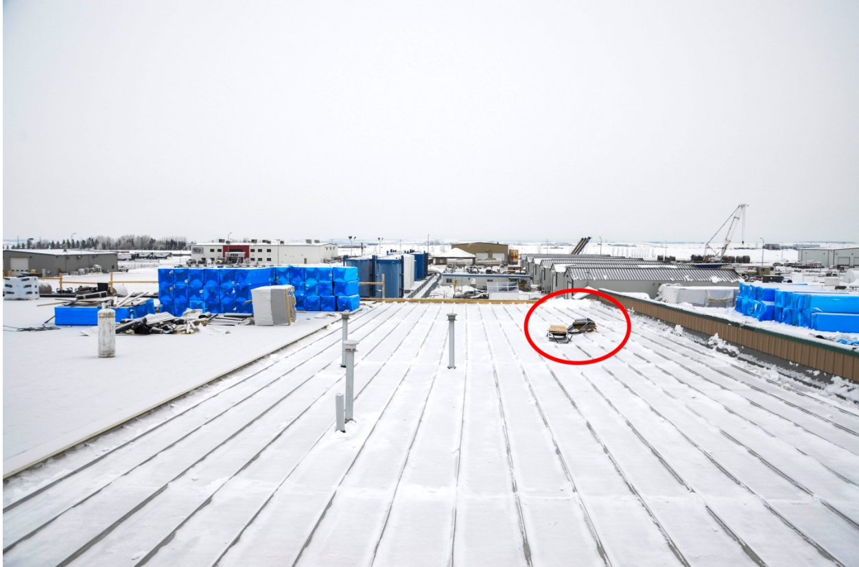
Figure 3. This is looking to the north side of the building. The red circle indicates the shovels that the workers were using to remove the snow from the tin roof. This was not the original location of the shovels; they were stacked together after the incident. (Photo taken by OHS)
