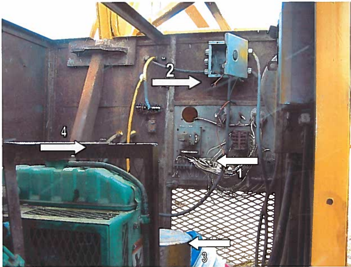
Photograph #5 Inside of the light tower looking from behind the Onan 4.0 GenSet generator diesel motor radiator to the electrical connections panel going from the step up ballasts to the metallic halide lights. Arrow #1 shows the live wire contacted by the Worker. Arrow #2 shows the neutral wire. Arrow #3 shows the ballast. Arrow #4 shows the metal radiator bracket the Worker layed on and grounded his self.
