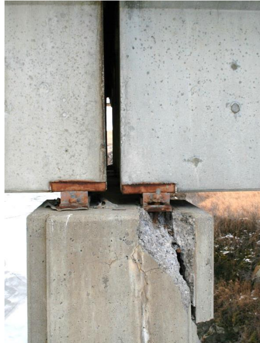
Figure 5: Concrete cap failure with girder drop in elevation.
