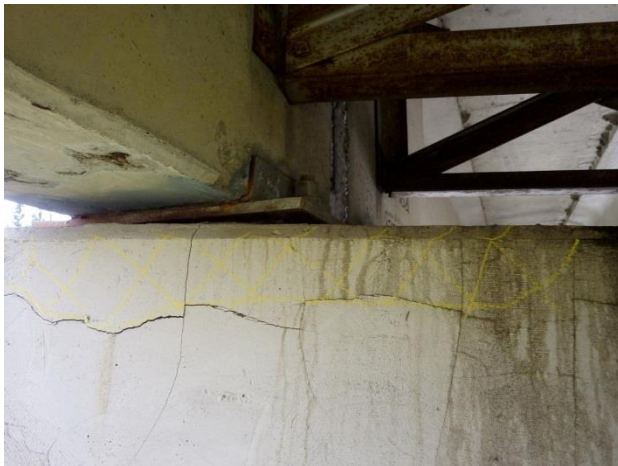
Figure 5: Wide cracks and concrete delamination in concrete S3G6 – P3. Pier cap and expansion bearing rated 3.
