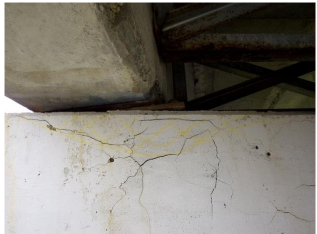
Figure 6: Wide cracks and delamination in bearing area of concrete cap at S2G1 - P2. Pier cap and fixed bearing rated 3.
