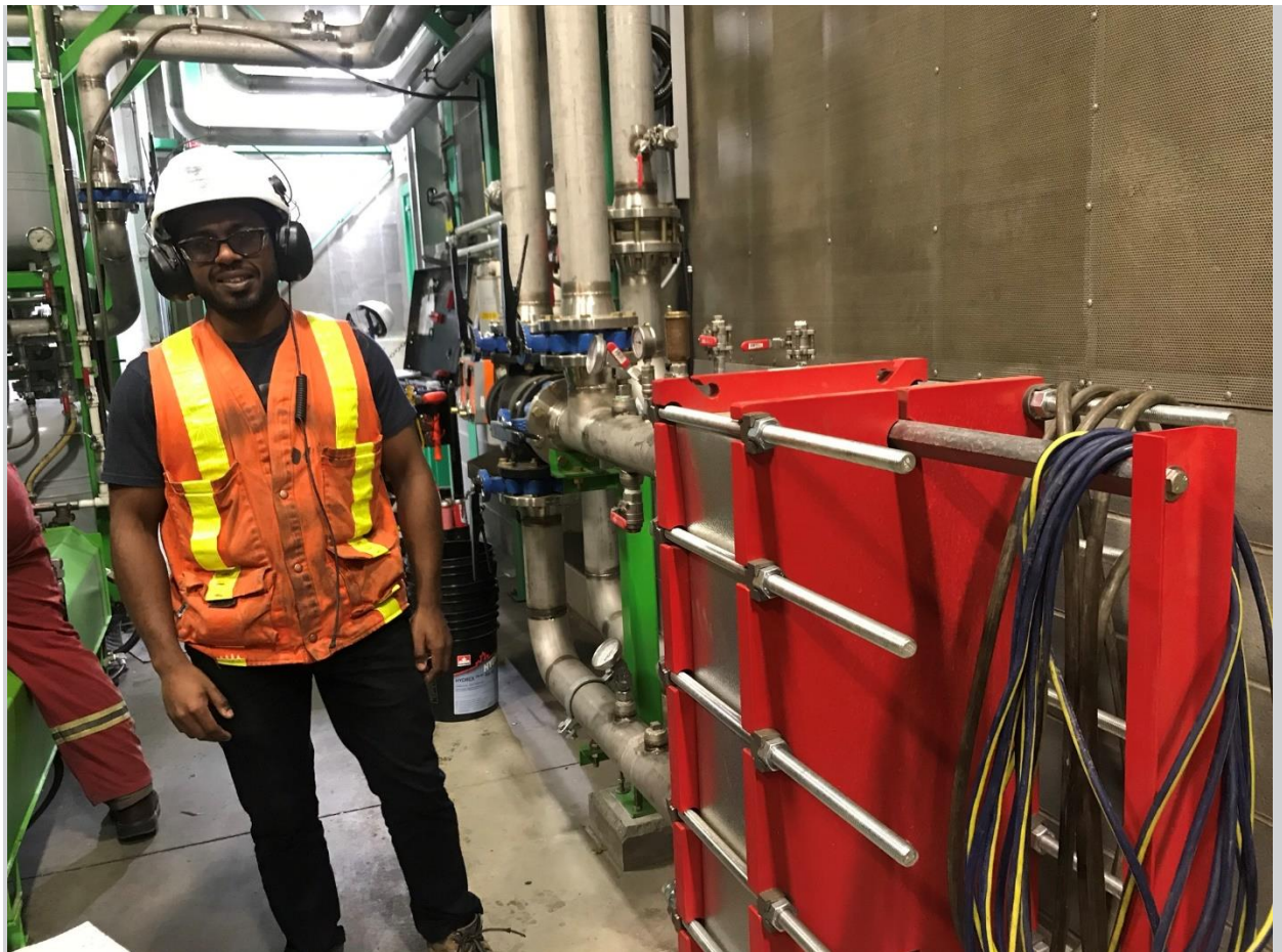
Stephen Newton, one of the energy champions, standing beside the heat exchangers.
