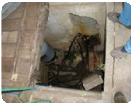
Figure 1: A typical well pit
