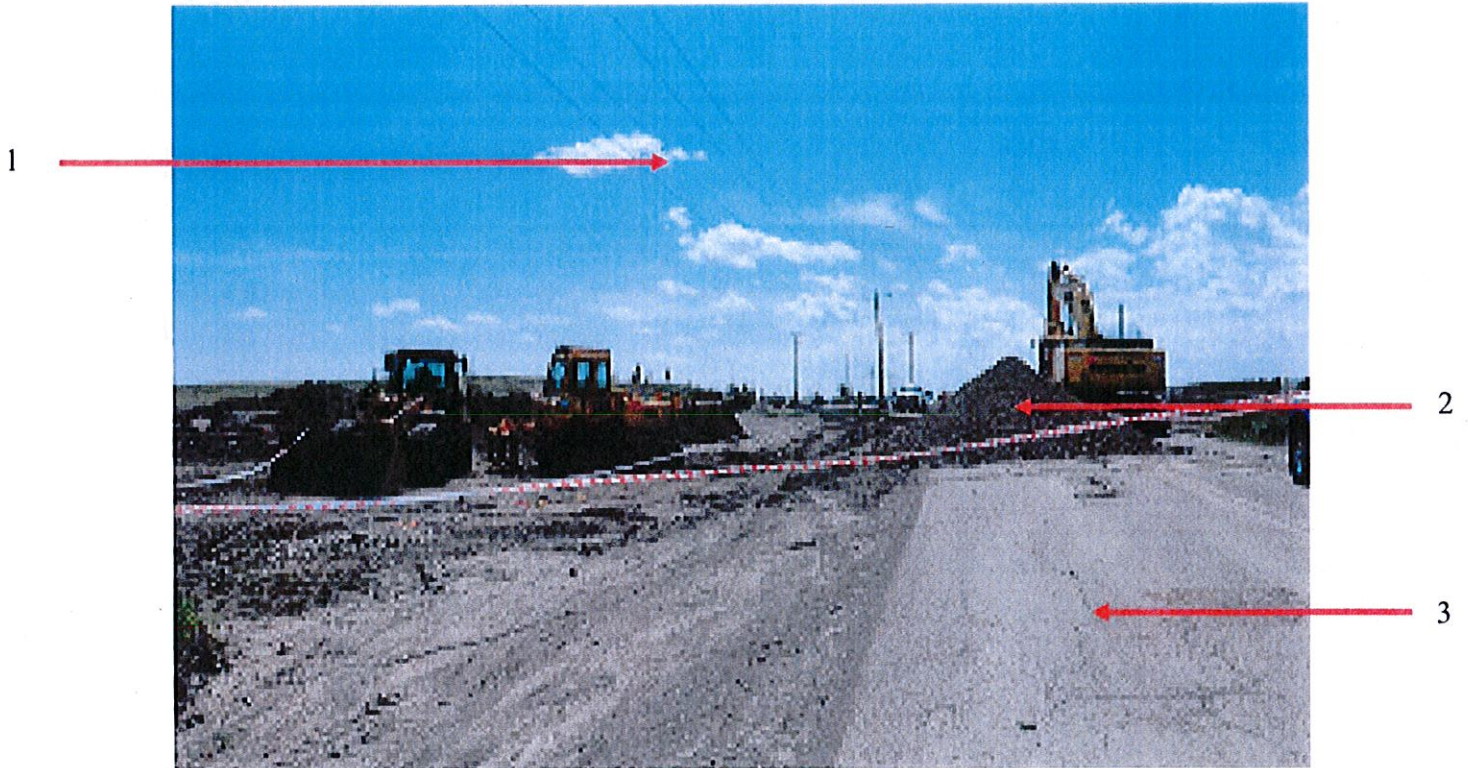
Photograph 2: Shows the view of the site of incident.
