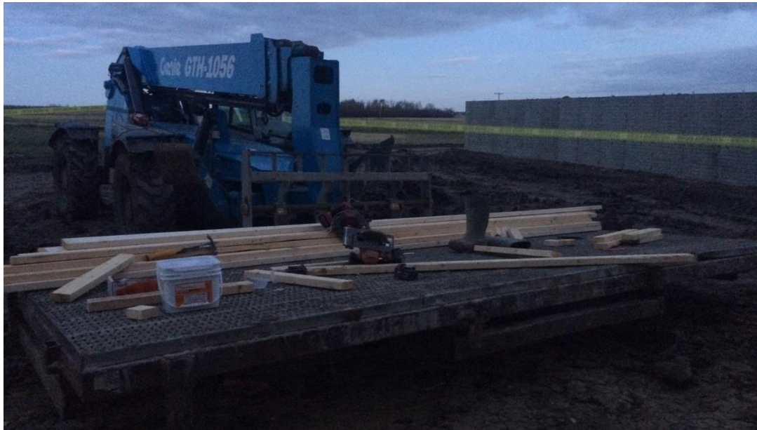
Figure 8. Genie telehandler work platform with tools and materials used to install fascia board on dairy barn.
