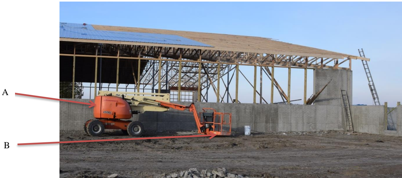
Figure 5. JLG telehandler with man basket attached. The JLG telehandler was located on the south side and east end of the dairy barn at the time of the incident.
