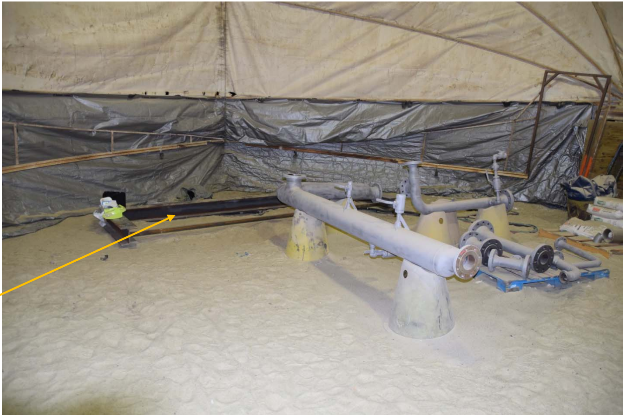
Figure 4. Sandblasting area showing the frame (indicated by arrow) the sandblaster/painter was working on as well as other work pieces supported on stands.
