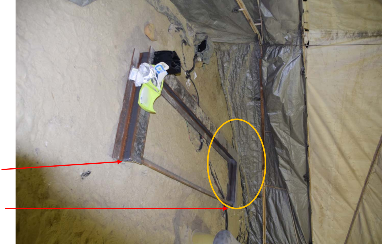
Figure 3. Frame section lying on ground in sandblasting area. Prior to the incident, the steel frame had been positioned in an upright manner on the ends of the short sections of the frame (indicated by arrows). The area in the circle showed indications of abrasive blasting on the surface.
