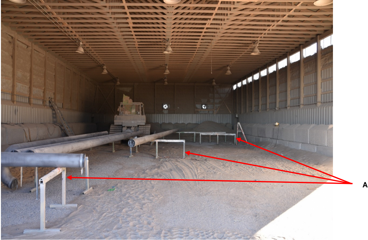
Figure 2. Post incident view of the bunks in the abrasive blasting building for pipe sections.
