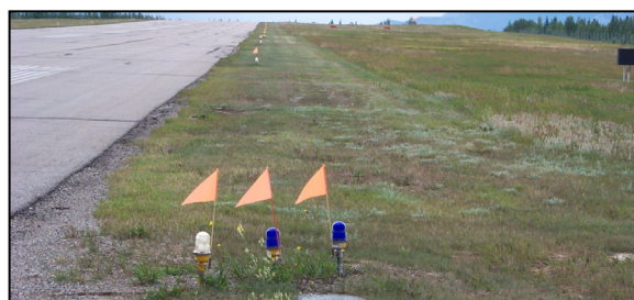
Runway (clear)/Taxiway (blue) Edgelighting System
