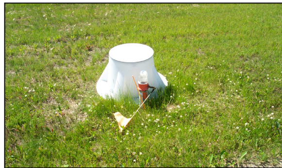
Runway Edgelight / Pullpit
