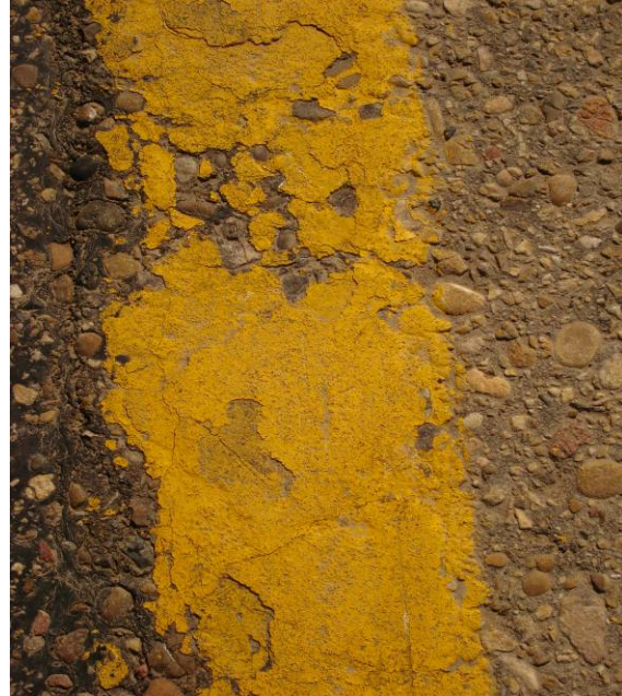
close-up, line has some minor chipping, otherwise in good shape
