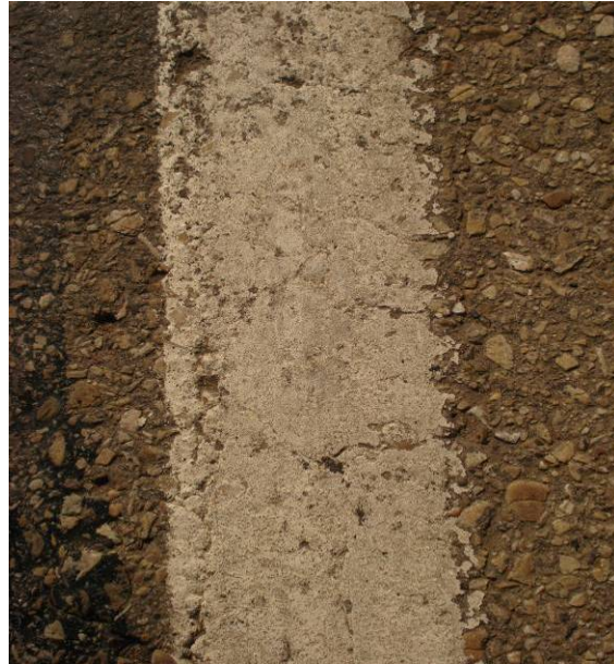
Close-up: durability is good, some minor chipping Observed, good glass bead retention
