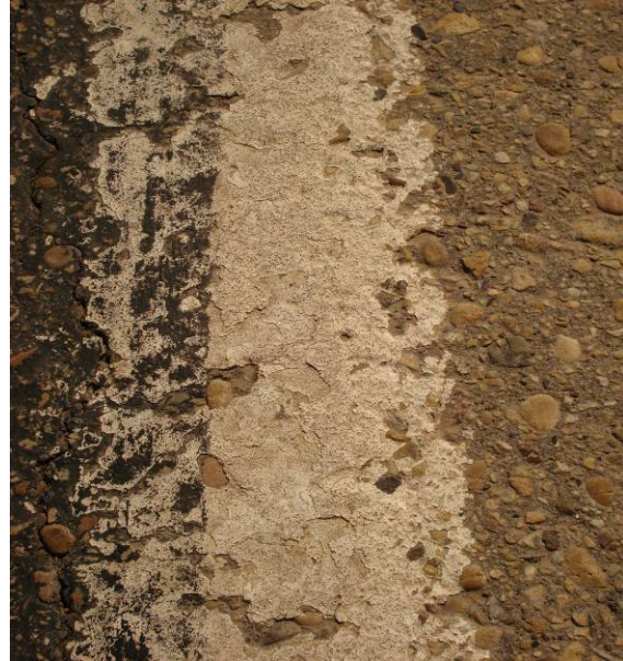
Close-up: durability is fair, some minor chipping observed, good glass bead retention
