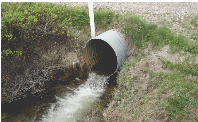
Hanging culvert that stops fish from moving into upstream habitat
