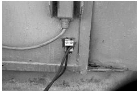
Note double metal-to-metal connection
