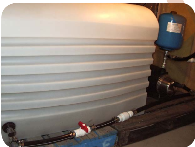
Figure 3: Tank and pump for low producing well
