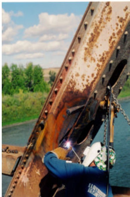
On compression members, cracks can be effectively repaired by welding. A bronze backing plate is used to separate built-up sections.
