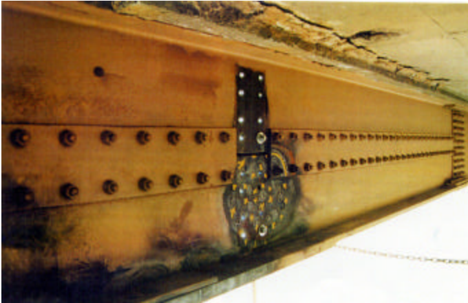
The top flange of a girder can become de-bonded or cracked at the deck interface from an impact event – the continuity and integrity need to be restored...
