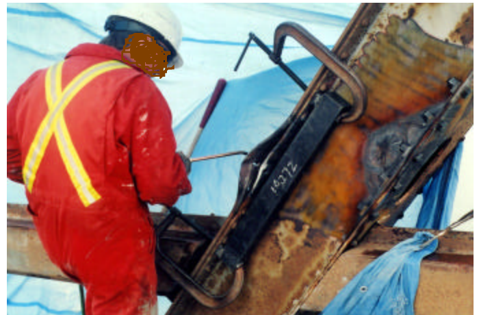
Heat straightening elements on a batterpost. Note the tarp being used to shelter from wind and cold.
