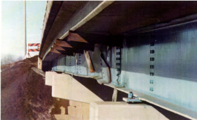
Severe structural damage events – such as with over-height impacts may warrant temporary deck support to keep the structure, or a lane in service...
