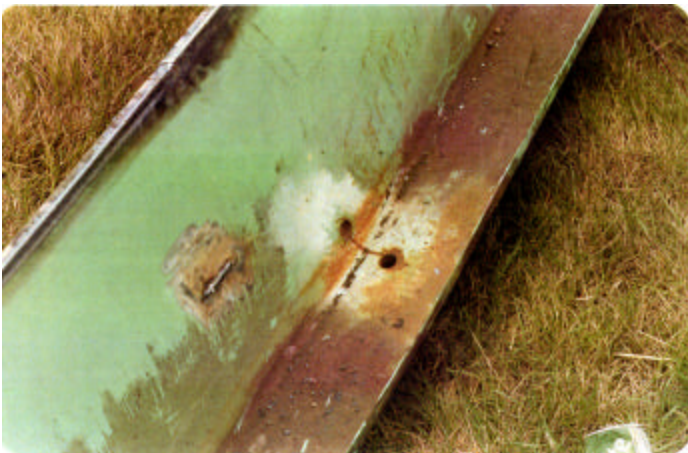
Drilling crack arrest holes in the flange and web can be effective in stopping the propagation of cracks – the far side of the flange is cracked across in the above photo.
