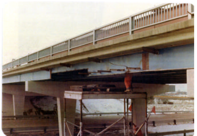
Girder cut-out operations can be performed in sections - allowing one lane of traffic to be maintained, and flowing at this stage of repair.
