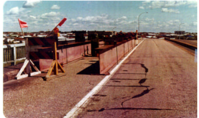
Temporary strongback deck support girders installed over damaged bridge girders – load transfer rods are installed at maximum 2.5 m spacing.
