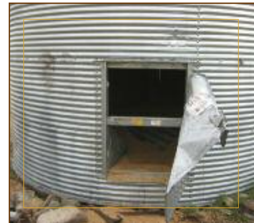
bear damage of graneries can be severe
