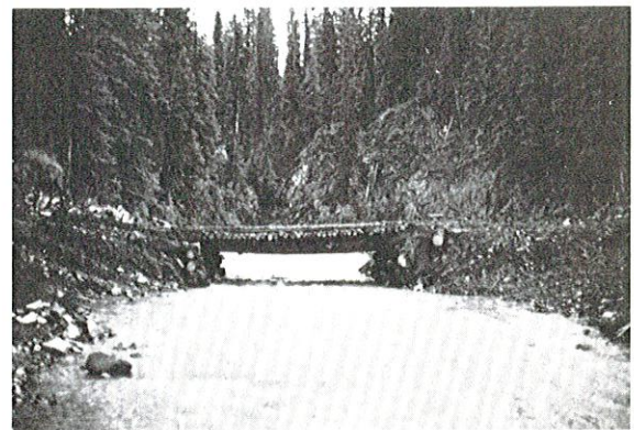
Photo 7. SIMPLE LOG STRINGER BRIDGE. Note absence of erosion control measures and that fording of the stream has also occurred.
