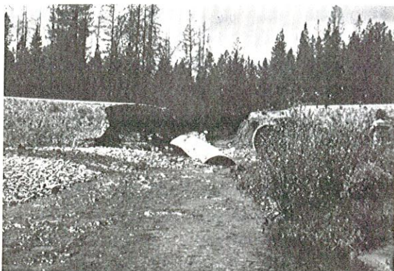
Photo 16. IMPROPERLY-DESIGNED AND INSTALLED CULVERT.
