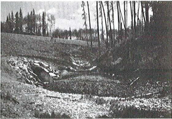
Photo 14. PROPERLY-INSTALLED CULVERT. A tapered culvert with large rock for riprap. Unfortunately, inadequate stabilization on slopes and fill resulted in heavy erosion into the stream channel.
