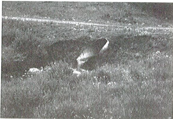
Photo 15. HANGING CULVERT. Cutback of the streambanks and road bed has occurred and obstructs fish passage upstream.
