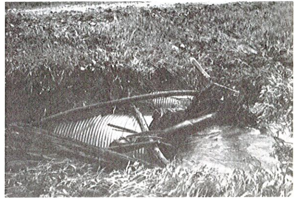
Photo 19. OBSTRUCTED CULVERTS. Inadequate maintenance allowed blockage by debris and sediment. Back flooding occurred and washed out portions of the road at the inlet and outlet ends. Four culverts are located at this site of which only two are visible.
