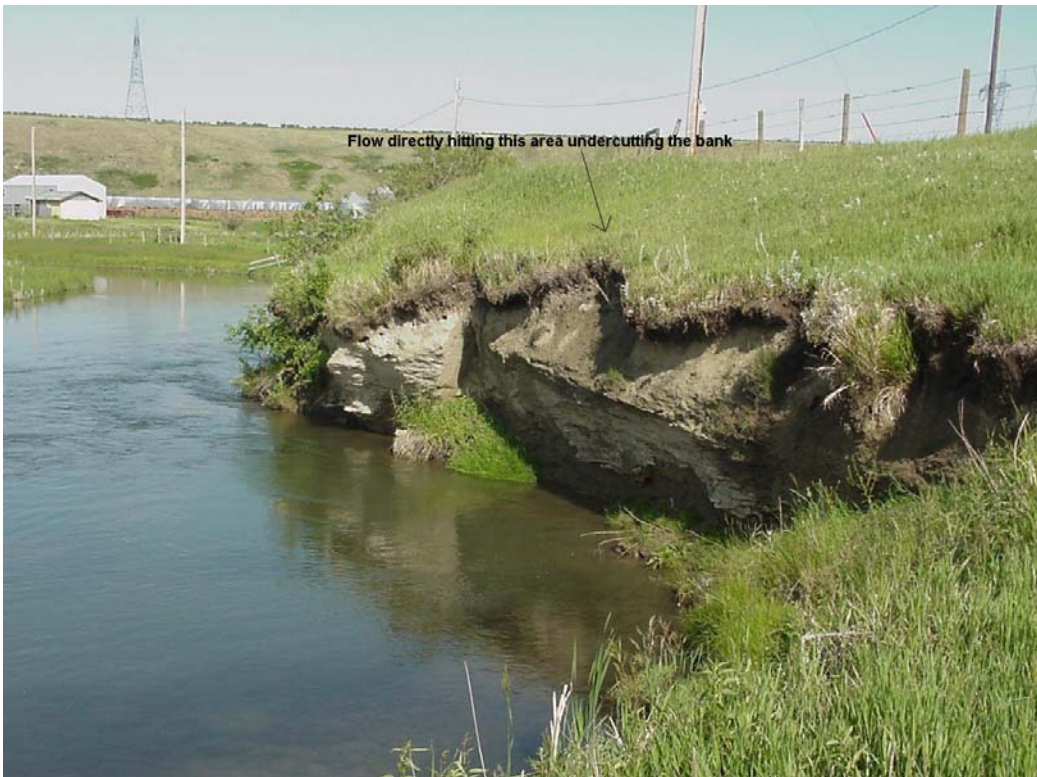
Figure 37. Erosion along Little Bow River between Highway 2 and 168 St.
