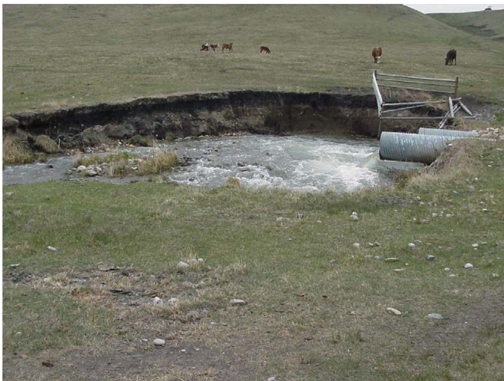
Figure 30. Eroding bank downstream from culvert near the owner's residence.
