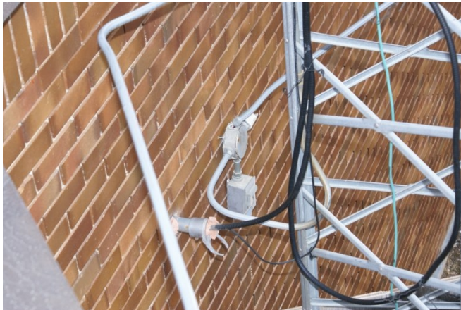
Photocell controlling roof mounted flood lights.
