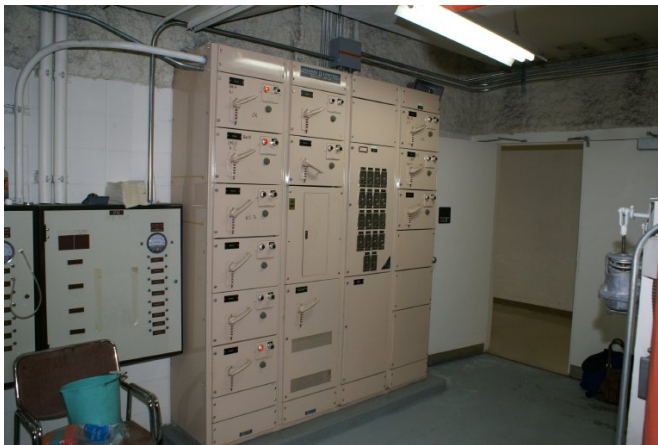
Motor Control Centre #MCC2
