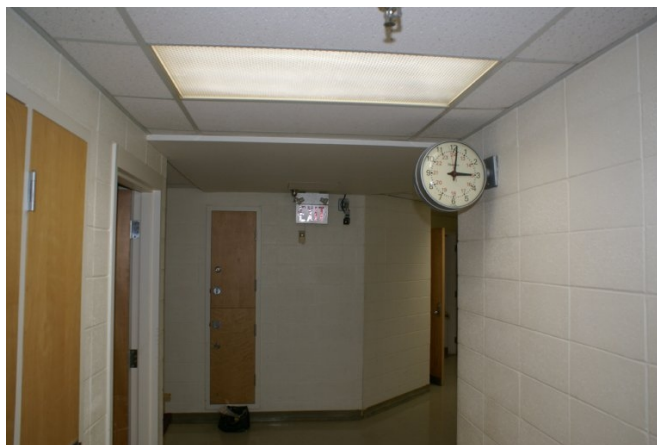
Typical corridor fluorescent light
