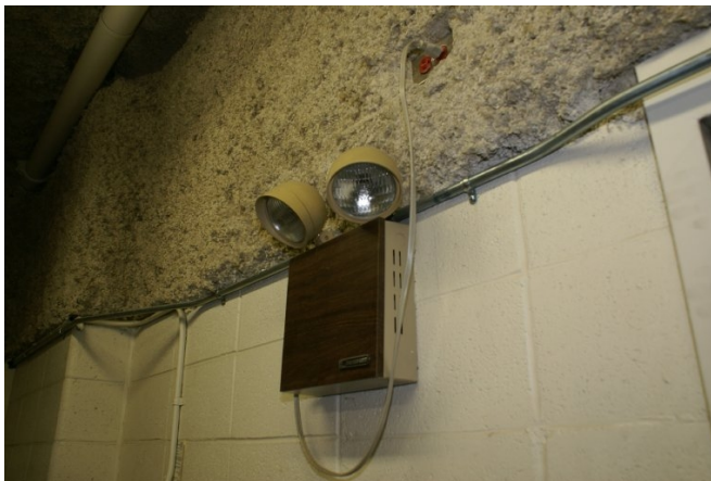
Emergency lighting battery pack in the generator room.
