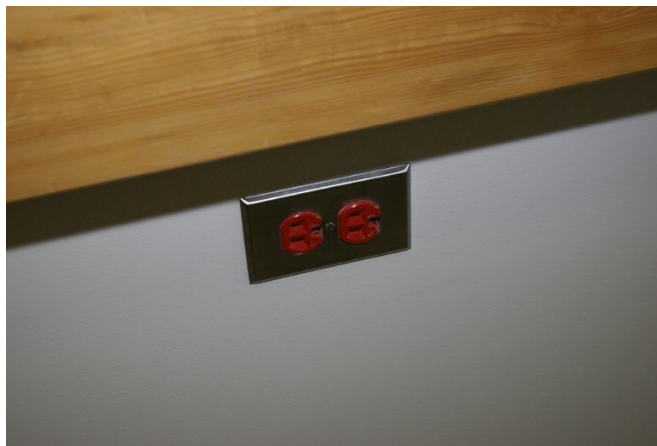
Typical Patient Room emergency receptacle
