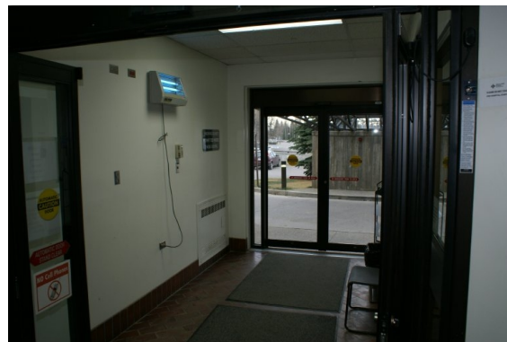
Fan coil unit and electric heater.
