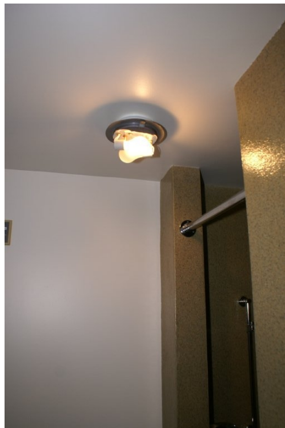
Incandescent dome light w/ missing lens
