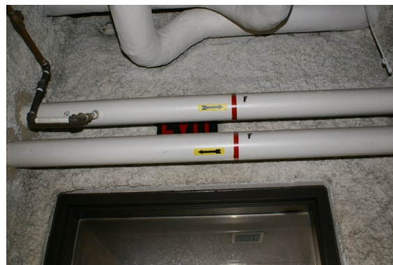
Exit sign blocked by mechanical piping.
