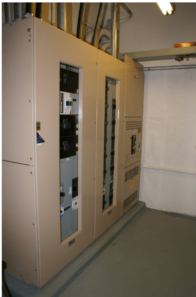
Main distribution panel
