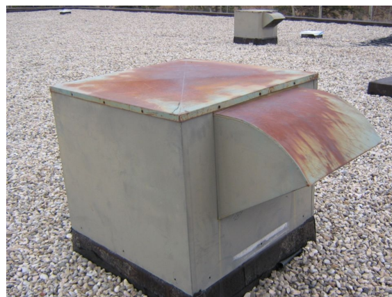
Roof mounted exhaust fan.
