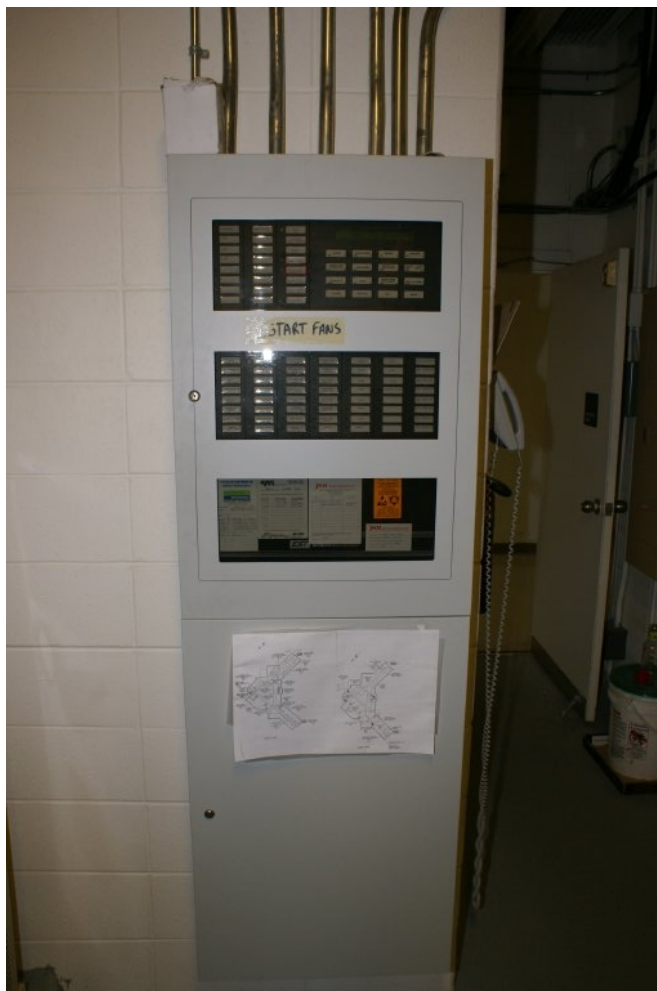
Edwards ESA2000 fire alarm control panel
