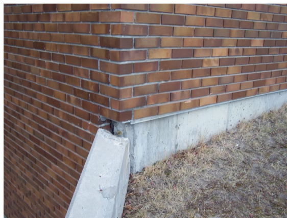
Retaining wall pulling away from building
