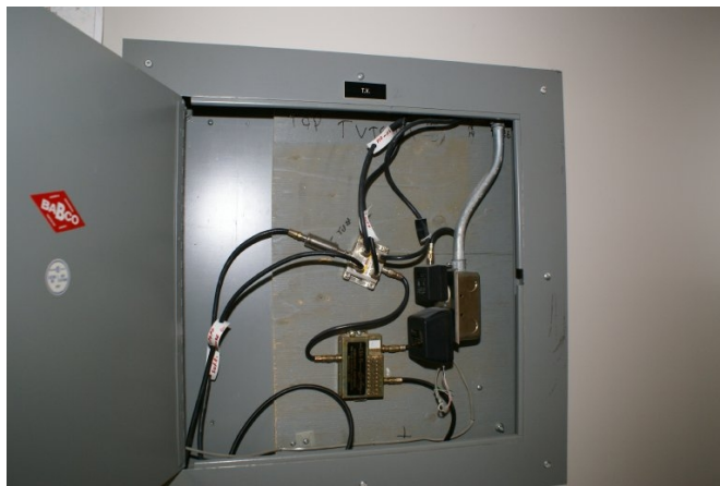
Sub-catv cabinet located on the upper floor.
