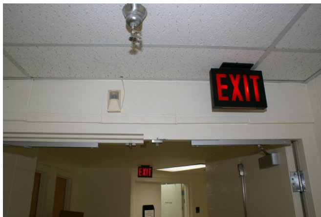
Typical incandescent exit sign.
