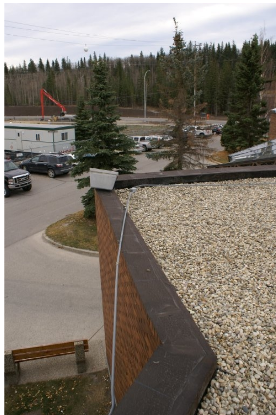
Exterior HPS flood light and damaged conduit
