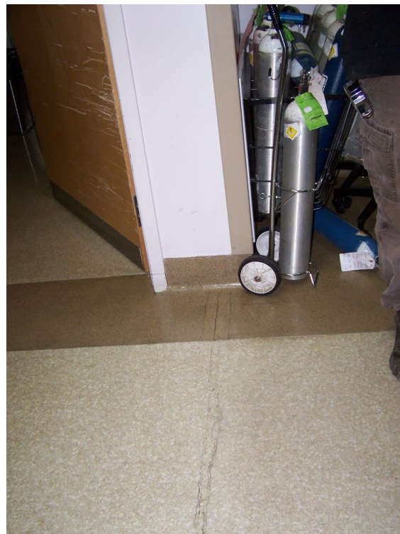
Failed control joint in floor
