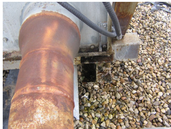
Corner that appeared to be leaking.
