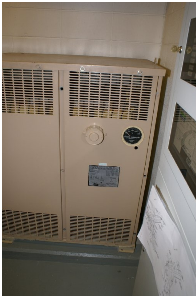
Federal Pioneer Transformer
