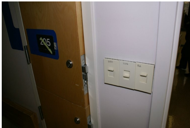
Typical patient room switches.
