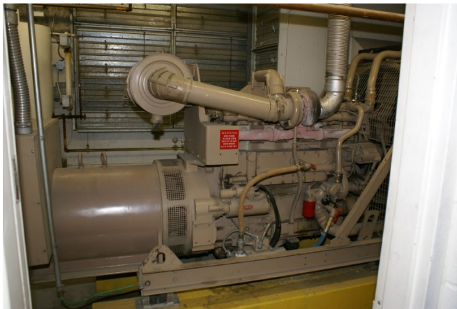
The diesel emergency generator
