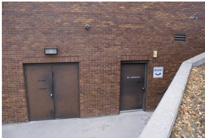
HPS wall pack fixture at Shipping & Receiving
