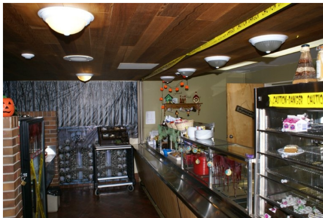
Incandescent dome lights in the Dining Area
