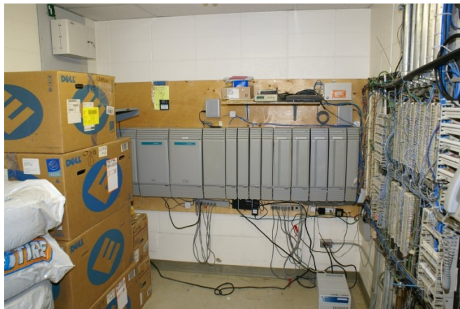
Main telephone demarcation and the Nortel Meridian PBX system
