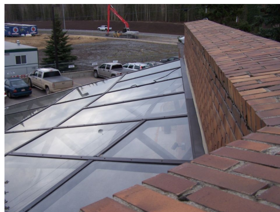
Caulk and sealing strips pulling away from glass panes
