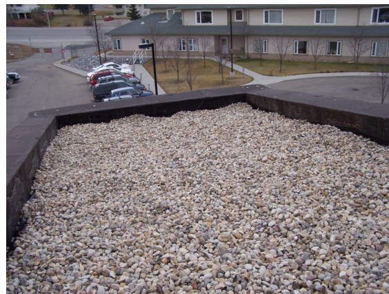
No capping on parapet walls
