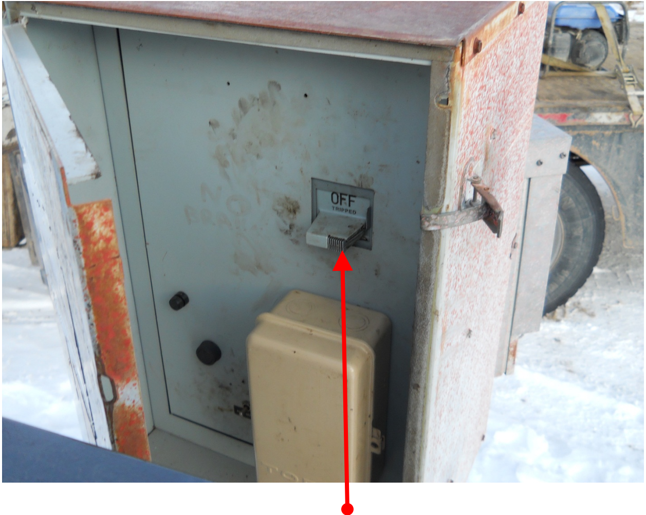
Pump jack electric motor disconnect switch in tripped position (off).
