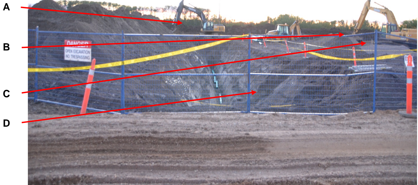
Figure 2. Photograph of work site, taken from the security fence which was behind securing fencing, showing piping, excavation and power mobile equipment.
