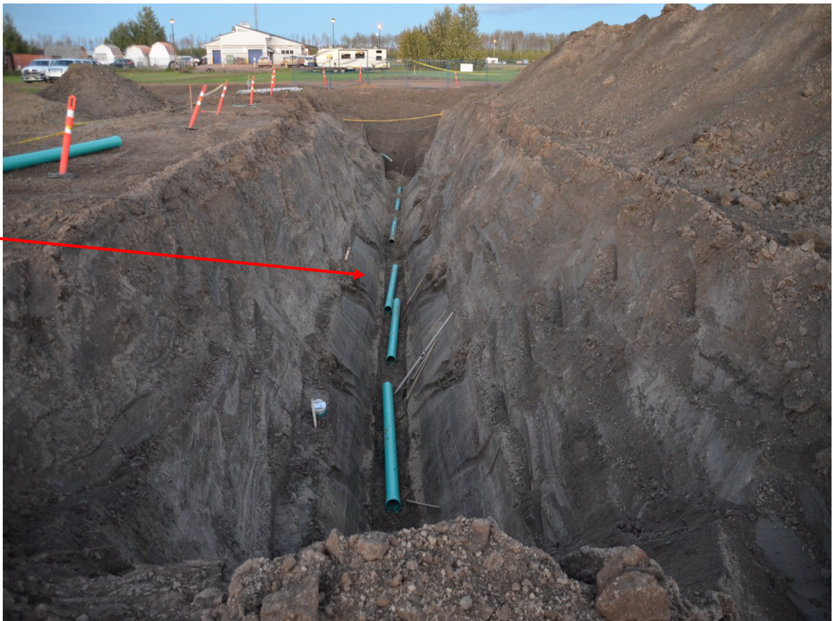
Figure 3. Photograph of the excavation where PVC waste waterline was placed. A. Approximate location where the workers were positioned while connecting pipe.
