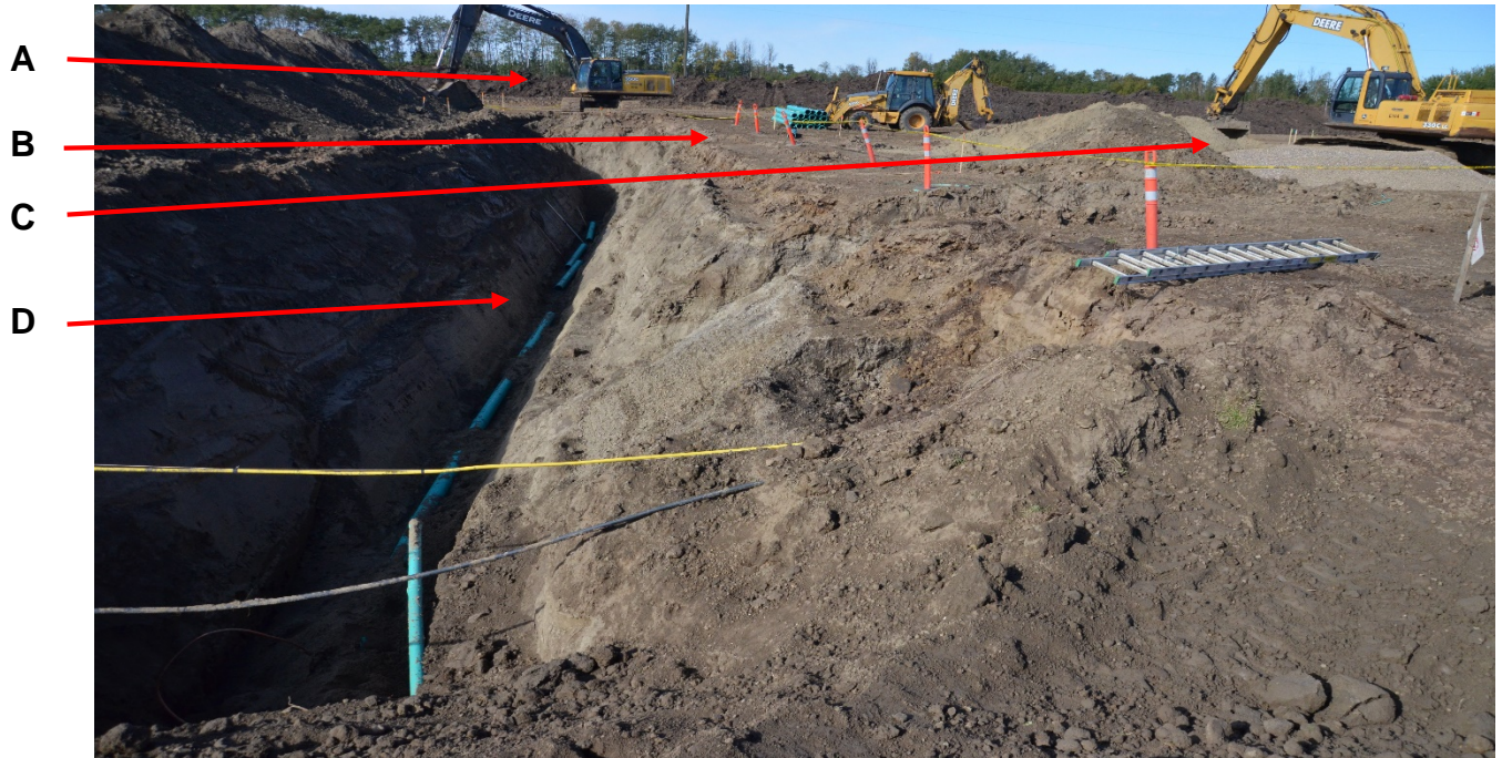
Figure 1. Photograph of the work site showing excavation, piping and power mobile equipment.
