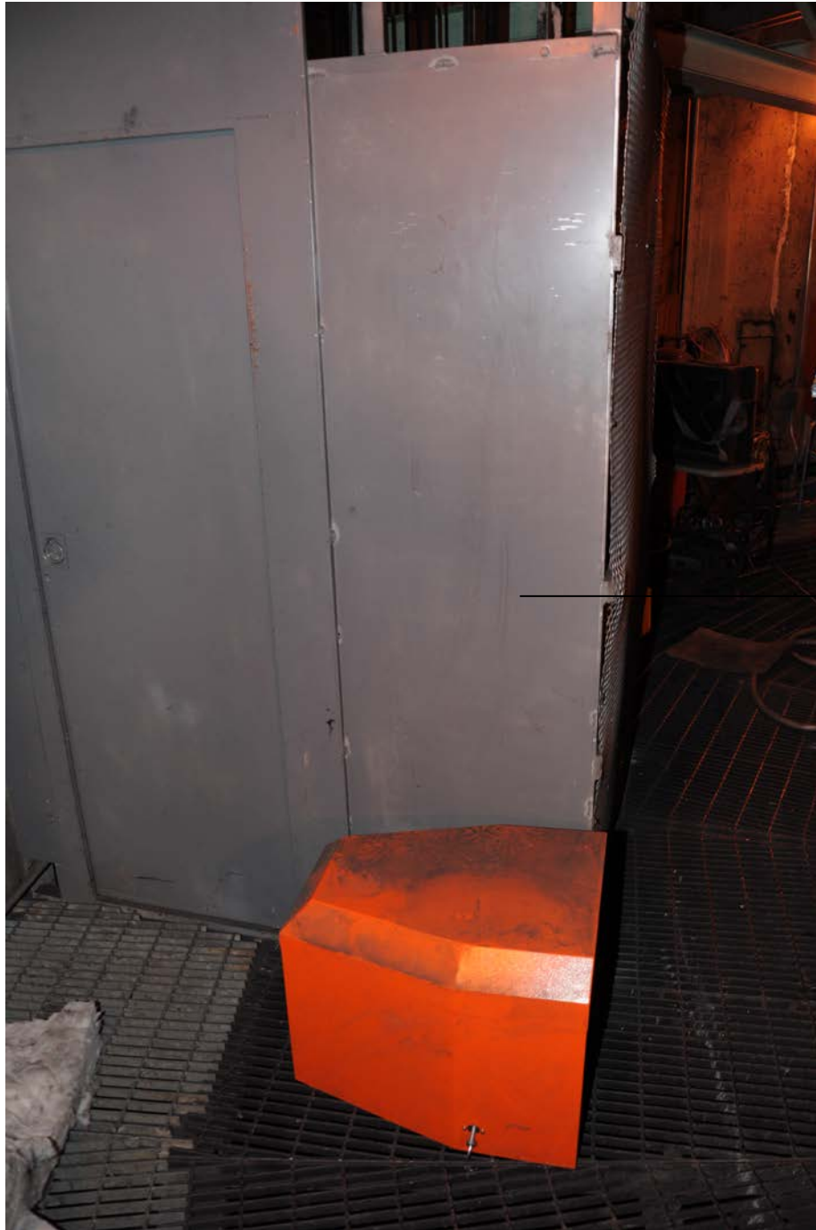
Photograph #3 Shows the upper hoistway as it was post-incident. Boot prints can be seen on the orange cover that had been placed next to the hoistway wall. 1 - Indicates the scuff marks on the hoistway wall.
