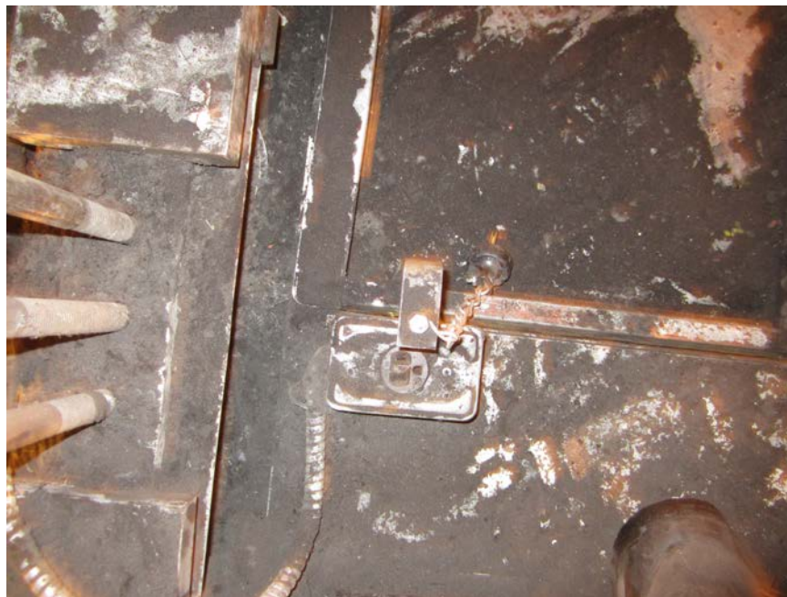
Photograph #9 Shows the emergency exit hatch safety switch on the roof of the elevator car as it existed at the time of the incident in both a closed (top) and open (bottom) position. Note the length of the chain connecting the plug to the hatch. Photo: [REDACTED]
