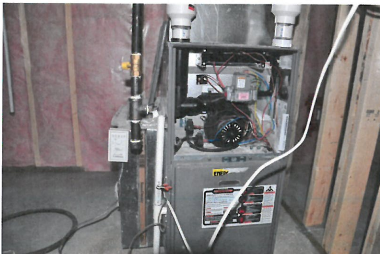
Exemplar of similar RUUD furnace installed in another residence.
