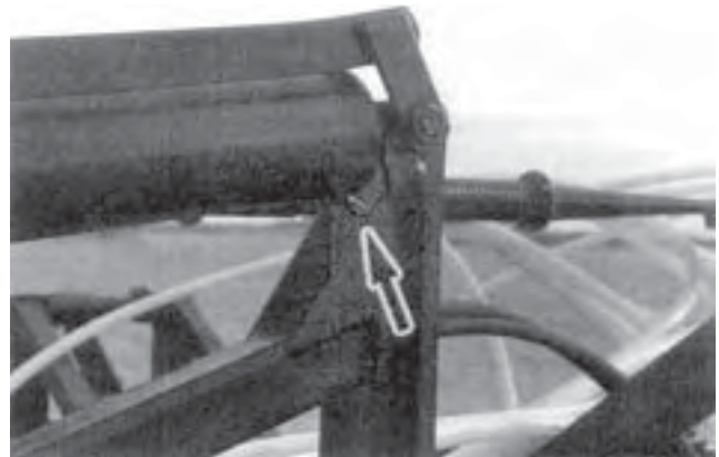
FIGURE 10. Cracked wing lift truss support.
