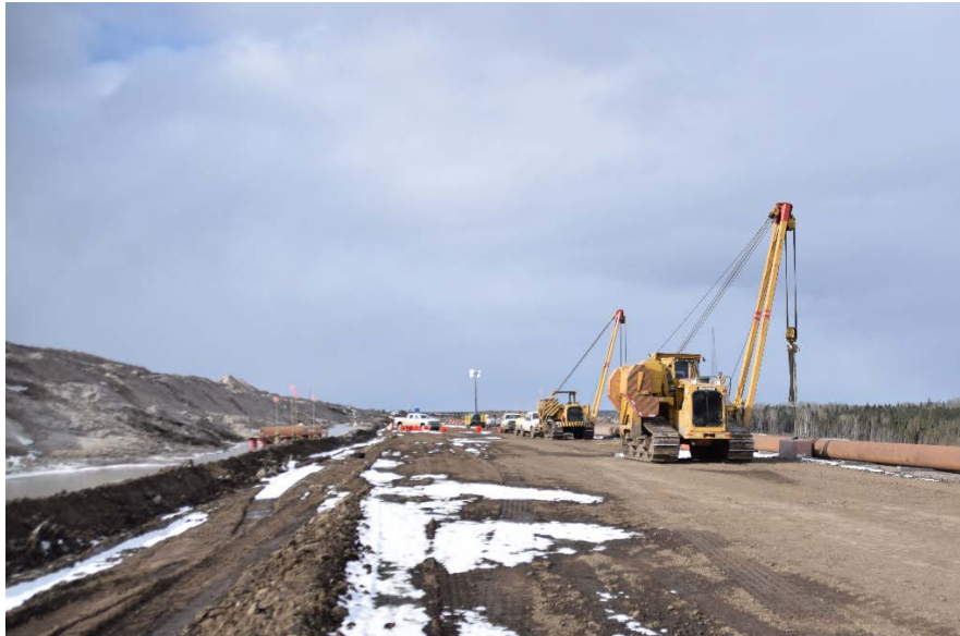
Figure 2. The work area where the incident occurred, point F in the aforementioned satellite image.
