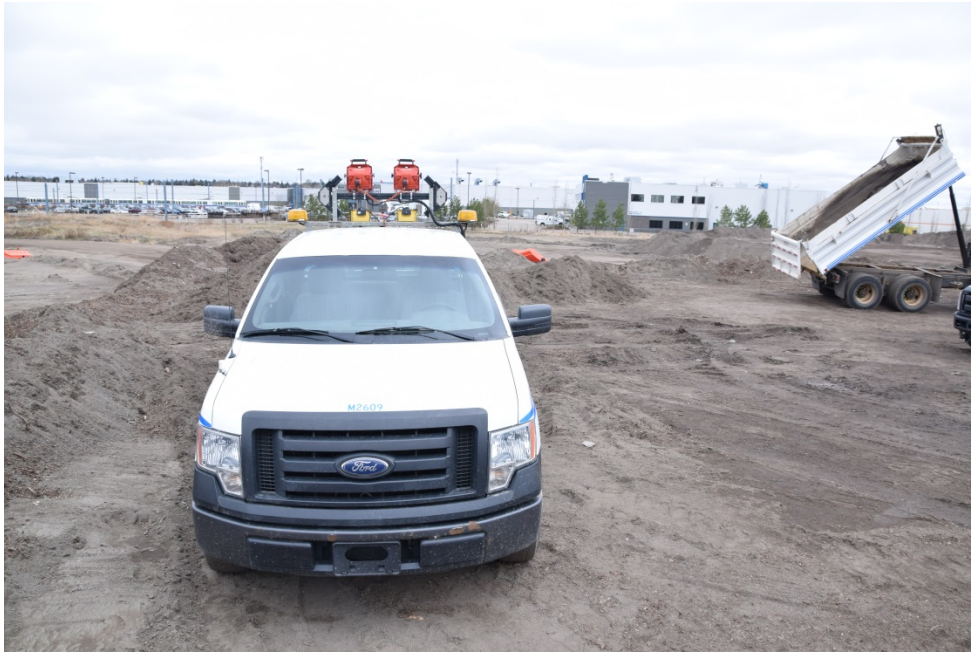
Figure 2. Truck was used to hold the lighting and generator for the worksite.
