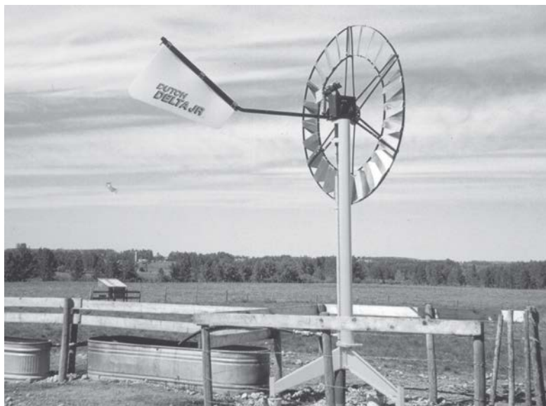
Figure 5-17 Wind-powered Pumping System
