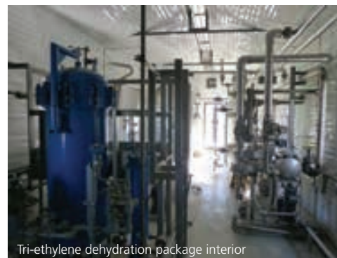
Tri-ethylene dehydration package interior
